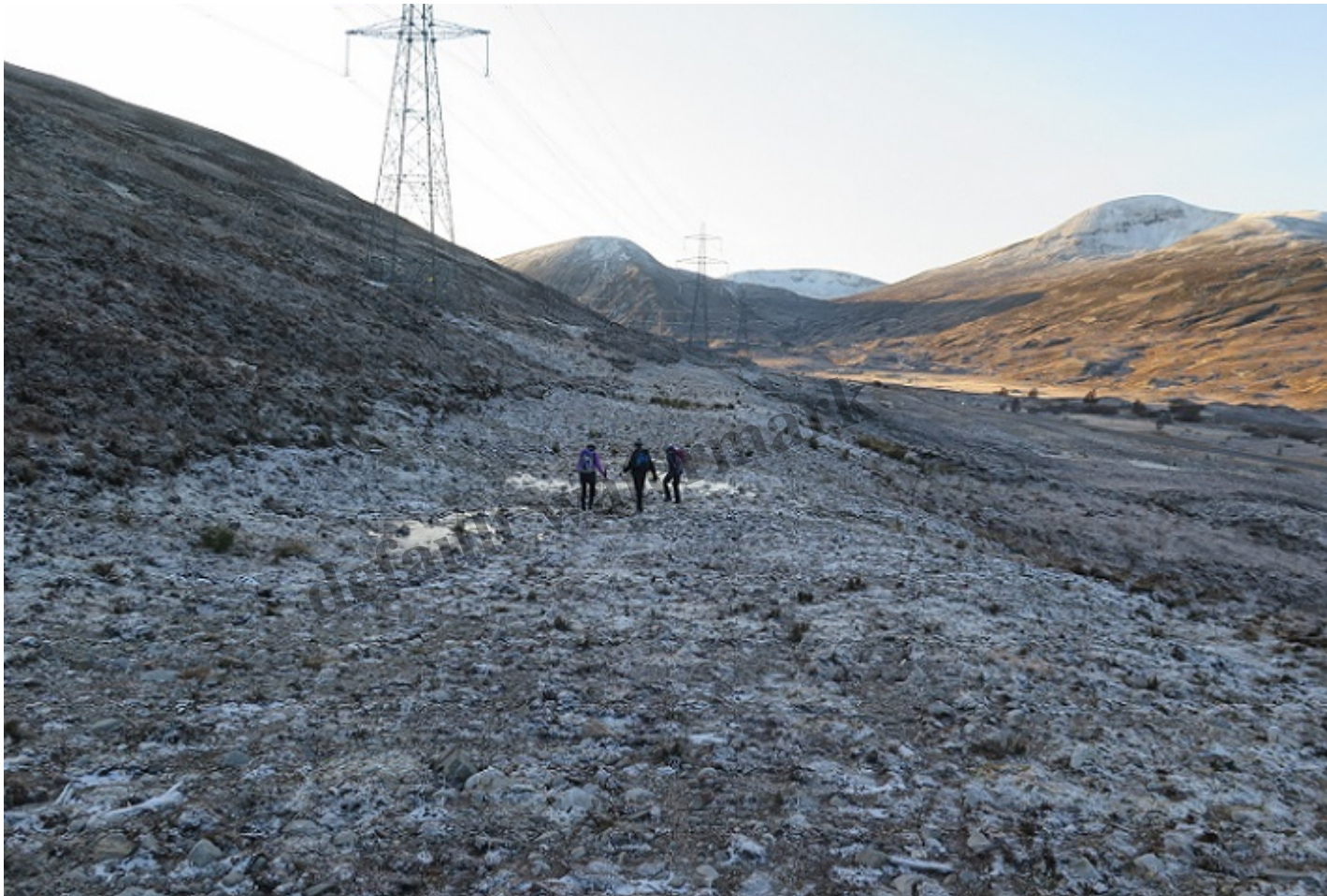
The unrestored powerline constructions track 1st December 2019. Photo credit Dave Morris
