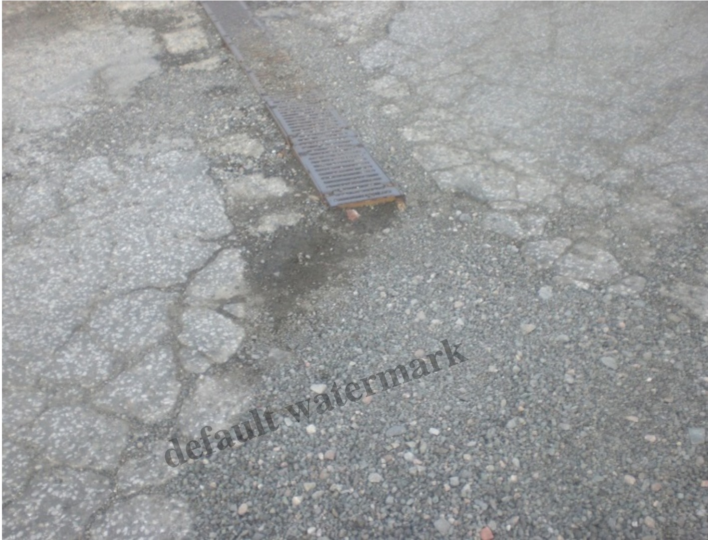
Broken drainage channel cover. Photo credit Alan Bratney.
