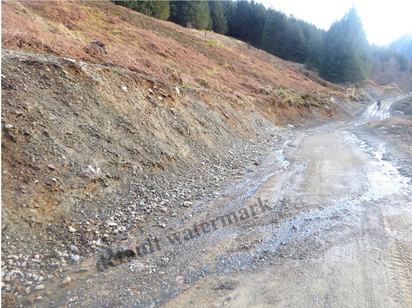
Steep instability and no sign of geotextile matting
