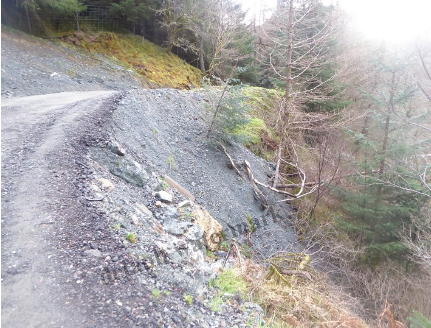
Bare edge of track eroding down towards the burn below – note the old abandoned concrete culvert
