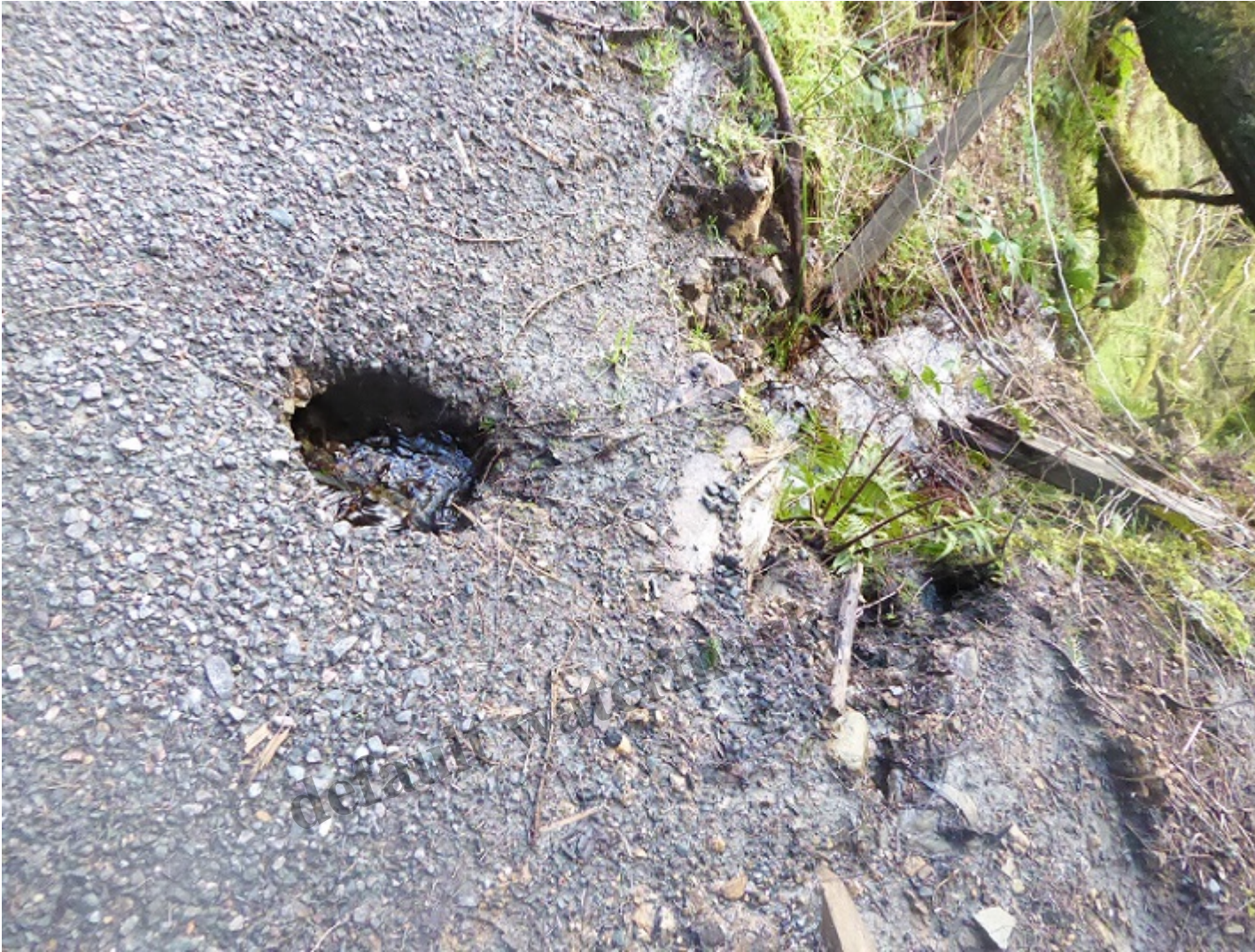
Road surface eroding from below
