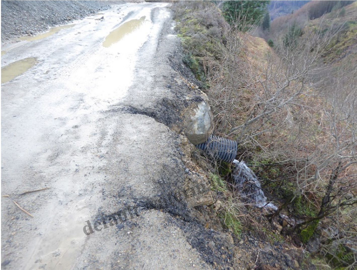
Culvert and road edge at high risk of collapse
