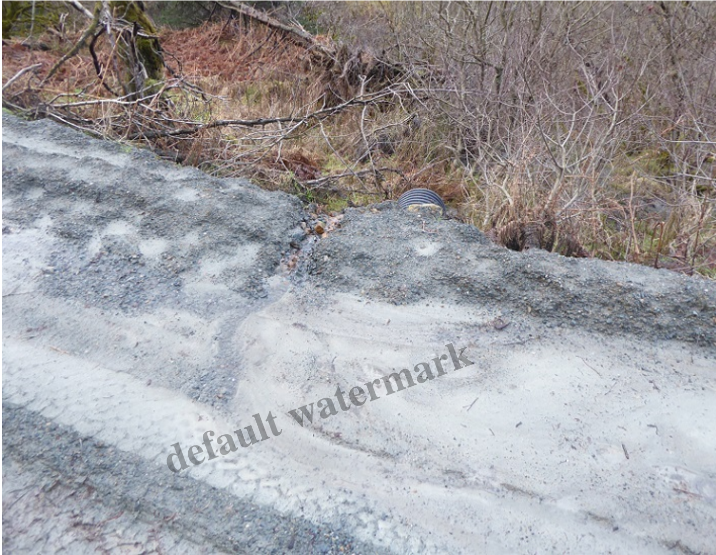
Another culvert likely to fail
