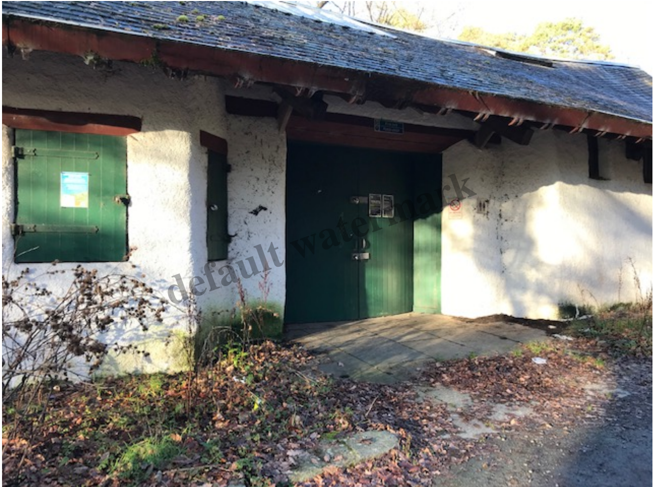
The LLTNPA toilets at Rowardennan in January, locked up and in a state of disrepair. Photo credit anon.
