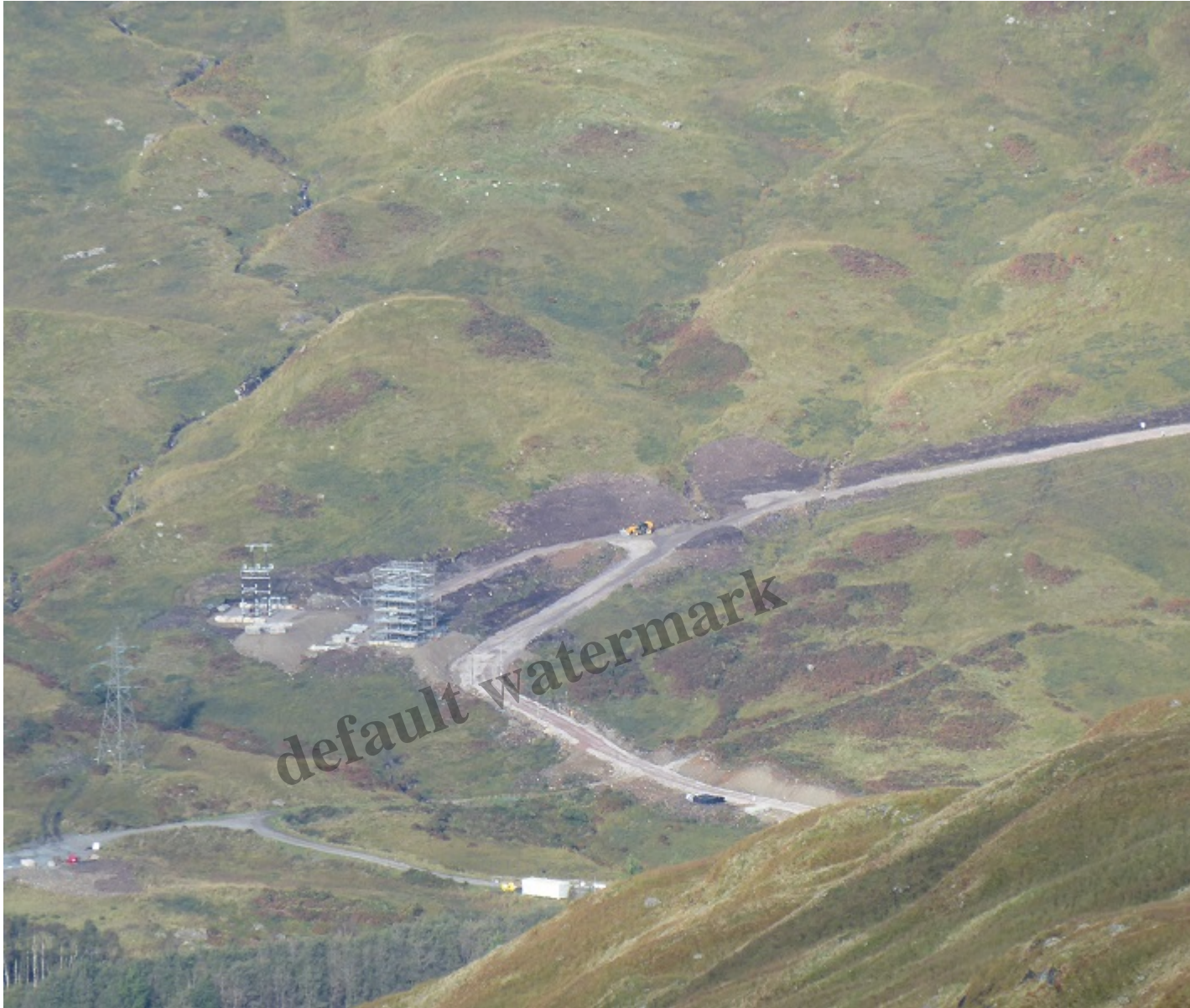
Close up of new temporary track and old and new towers above Derrydarroch
