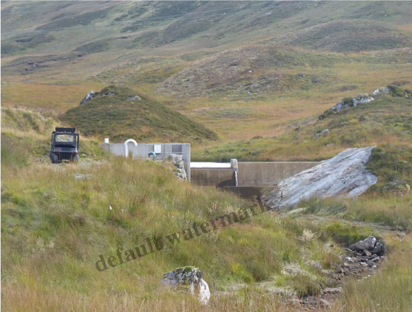
Second hydro intake, with pool behind and half empty burn below. Photo credit Louise Brimelow.
