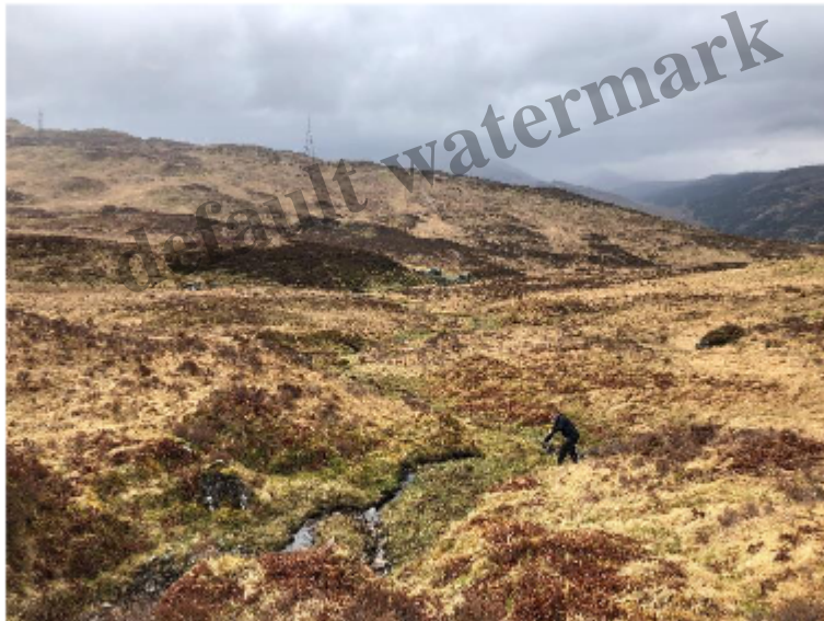
Figure 4: Looking from Intake G to the tie in with existing penstock pipeline at the vehicles.
