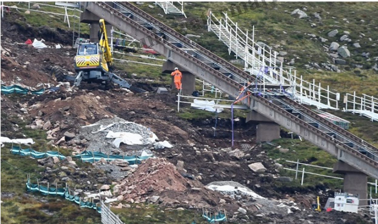
The sheer amount of the earthworks and imported materials provides evidence that the repairs are significantly greater than originally planned. Photo credit George Paton September 2021
