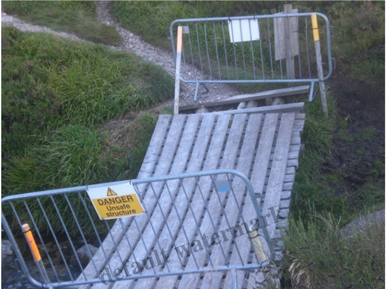
The bridge over the Allt na Ciste remains broken and prevents easy access to the East Ciste paths. Photo credit Alan Bratney.
