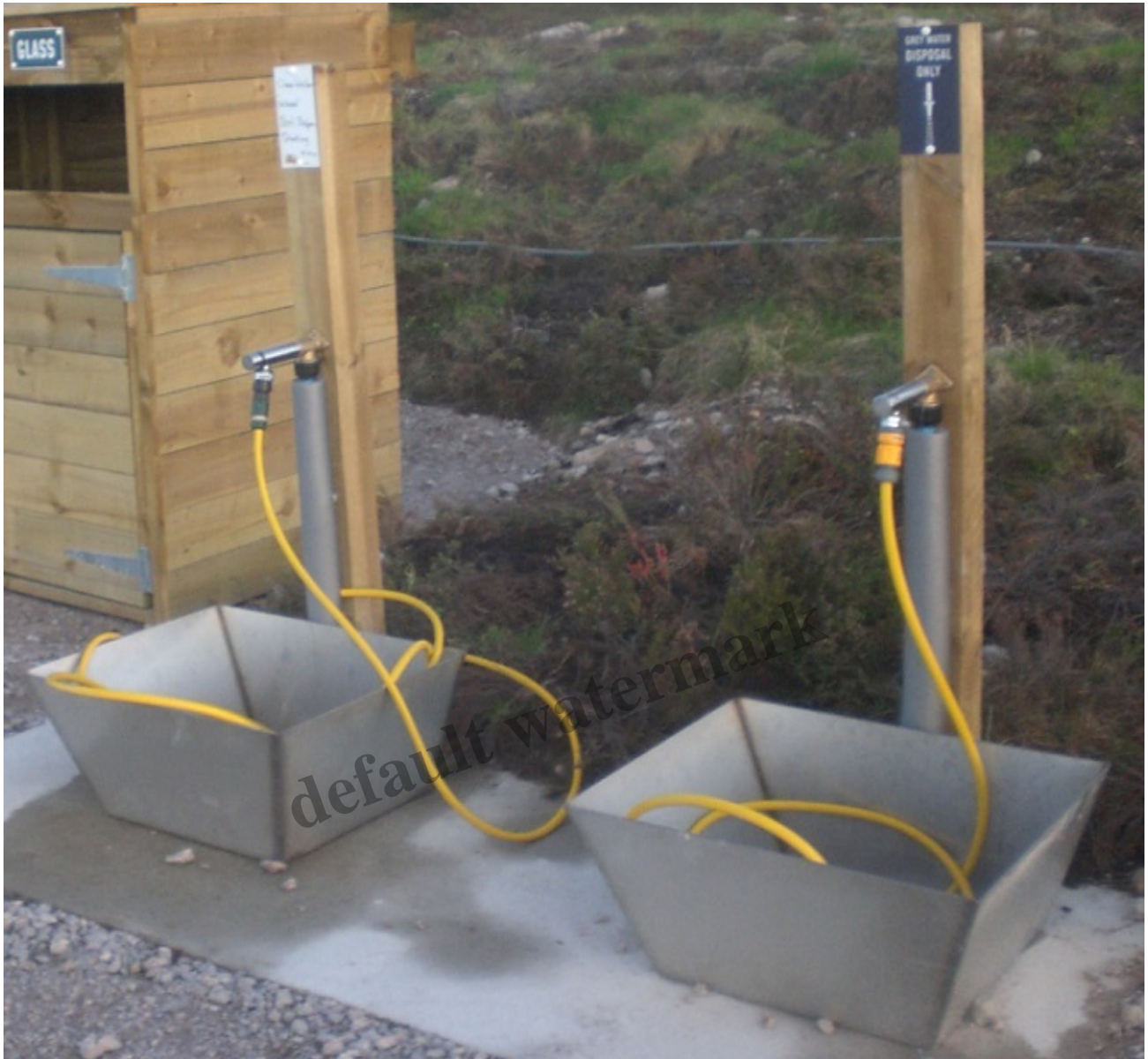
The “clean” water facility on the left, the grey water disposal facility on right
