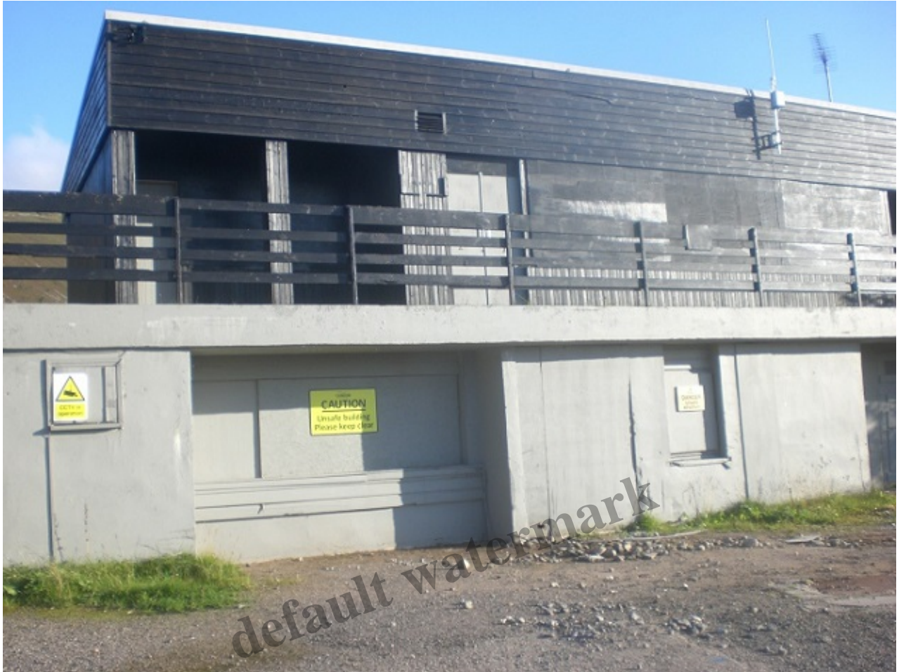
The Ciste base station building remains unsafe. Photo credit Alan Bratley.
