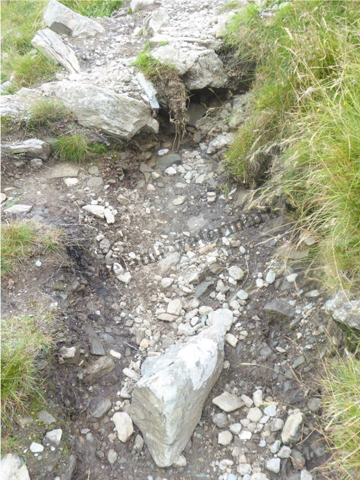
Note how the boulder in the foreground, which once formed a step, has been eroded out of the path.
