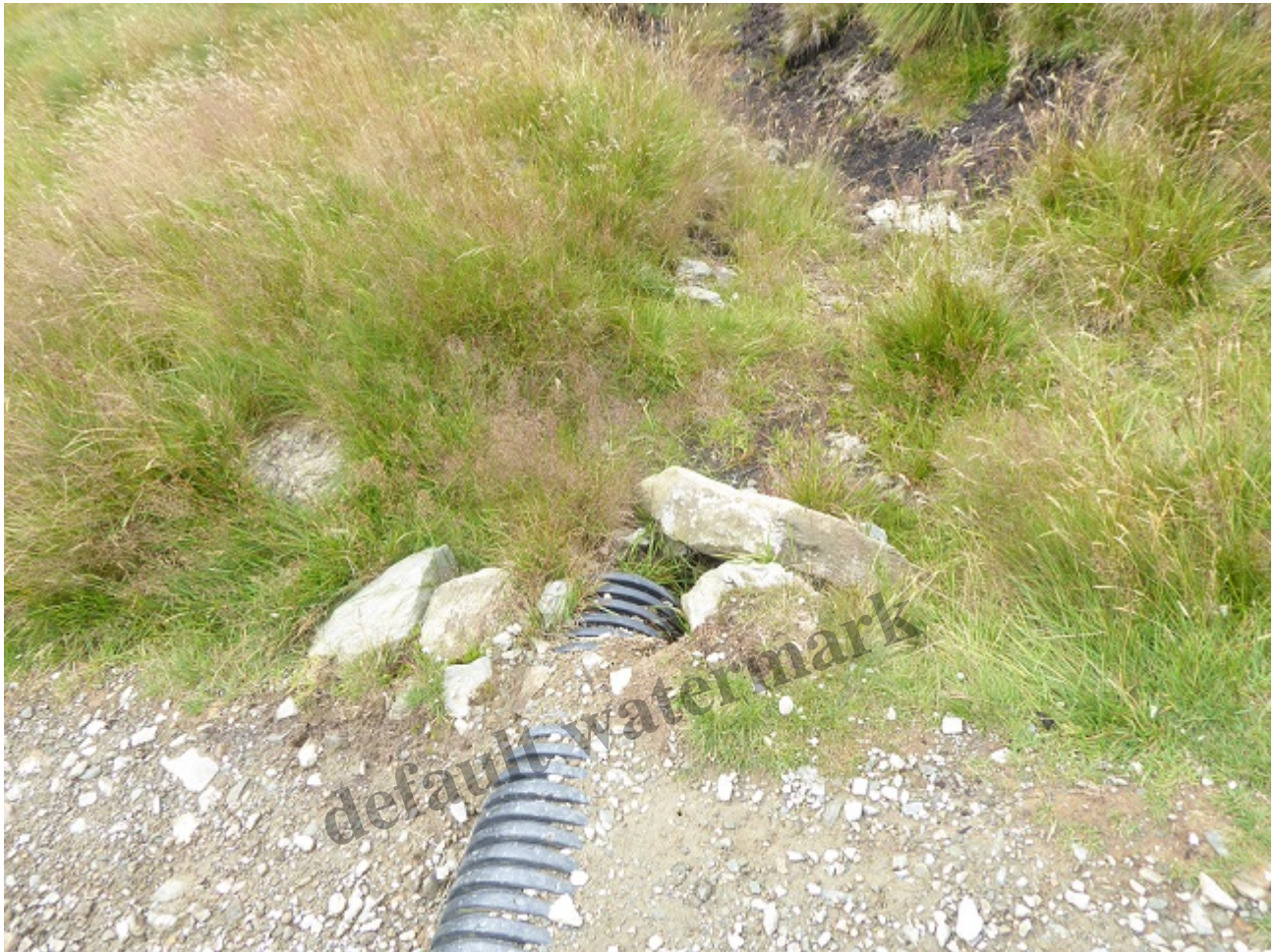
Exposed culvert with dislodged capping stone beyond. If it looks bad, it is bad!
