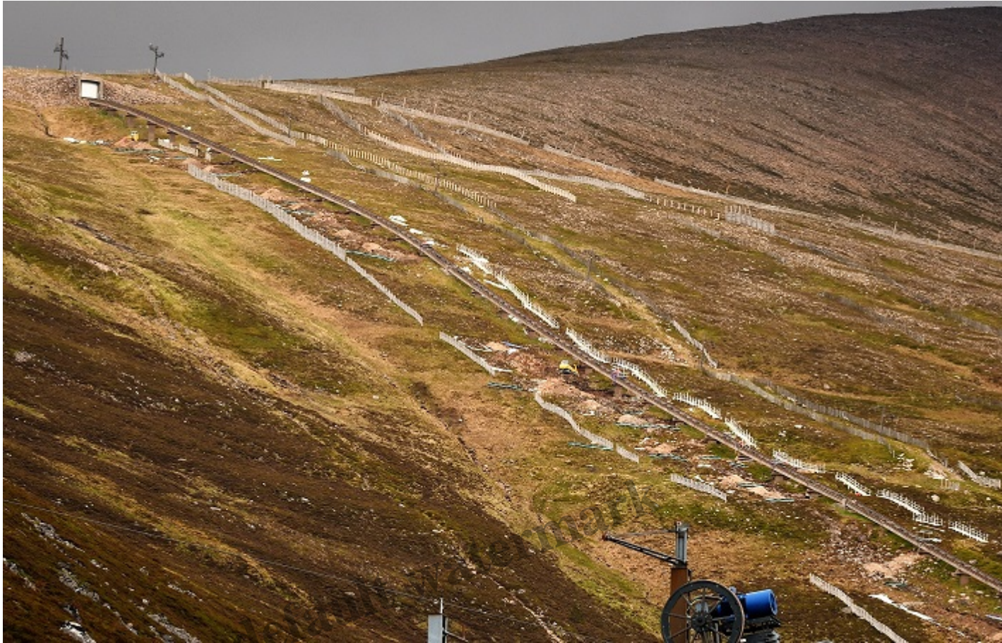
View of repair work above the mid-station to the funicular tunnel, top left, with sections of walkway in place on the far side of the funicular. Diggers are visible top left and centre. Photo credit George Paton m
