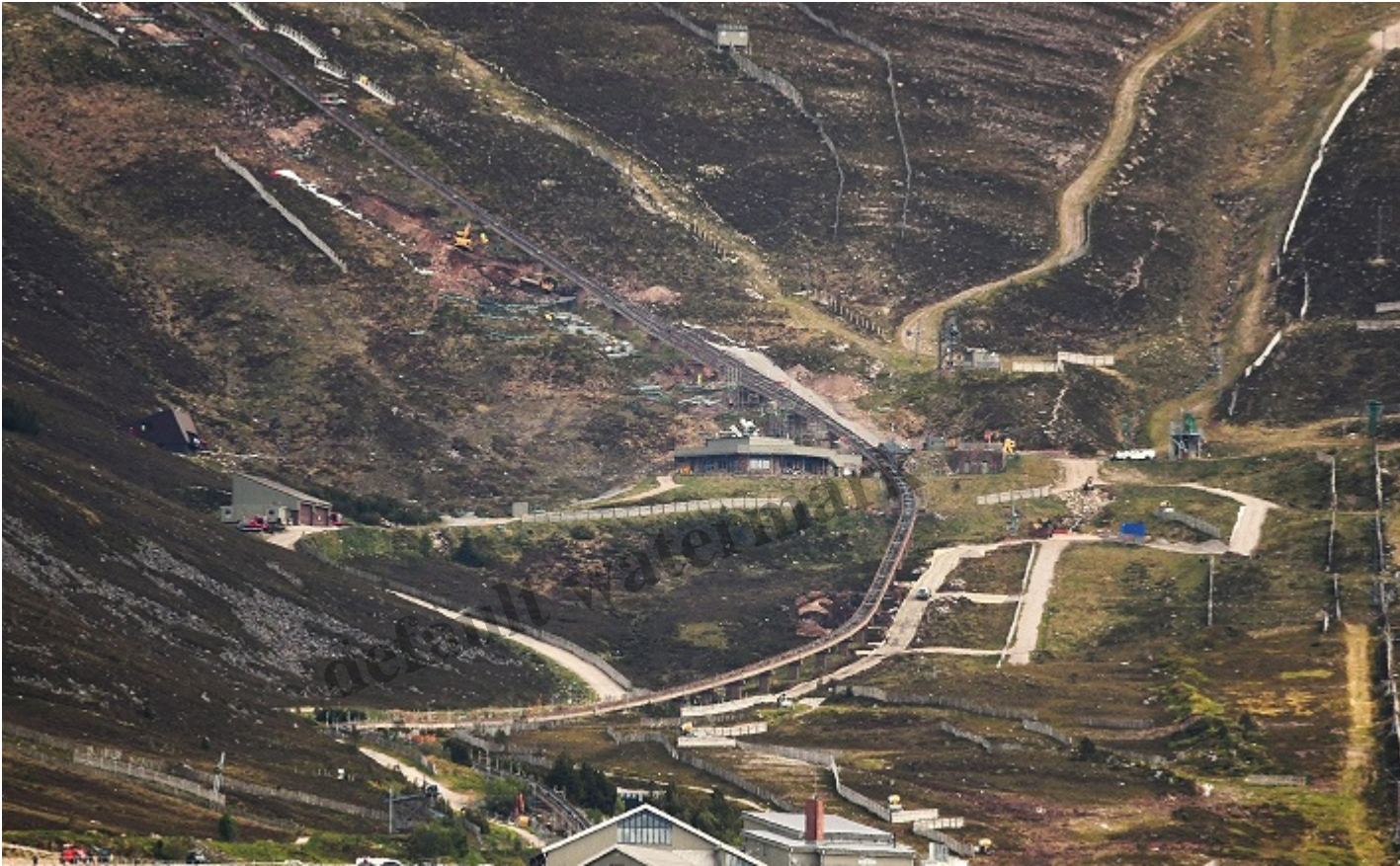
View of middle section of funicular repair work showing temporary access tracks on righthand side of track and extensive earthworks by and above the mid-station. Photo credit George Paton mid-June
