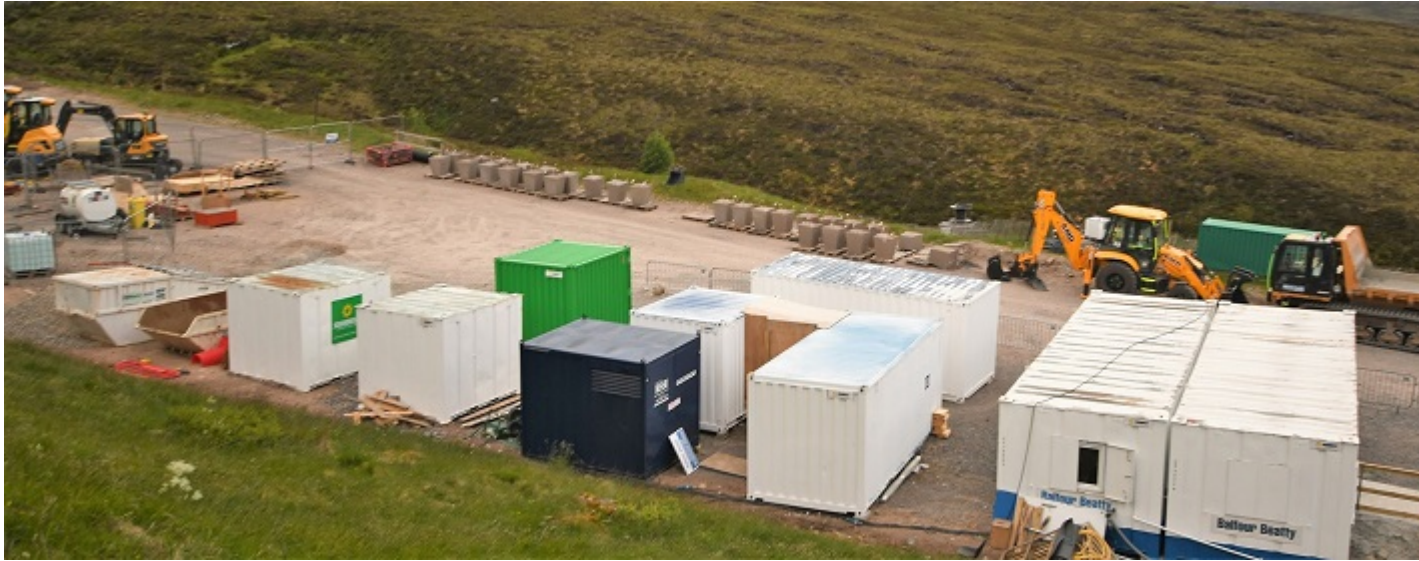
The western half of the lower Coire Cas car park is being used as a compound for the funicular repair. Photo Credit George Paton.
