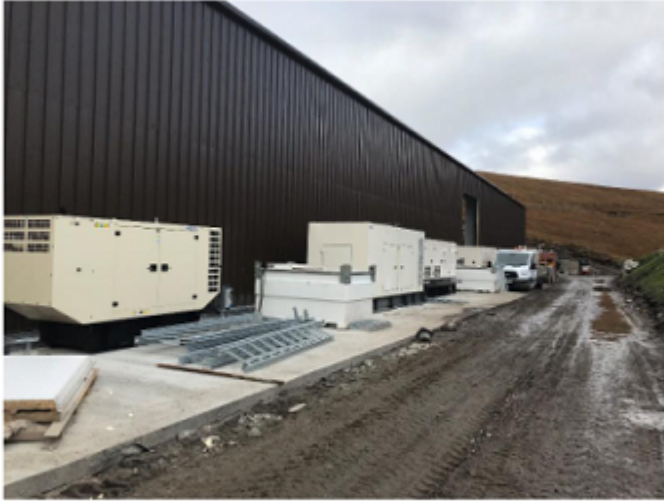
Plant Platform - Front of the processing building the area for Fuel storage tanks and generators (all generators are integrally bunded). Heavy duty protective barrier system to be installed
