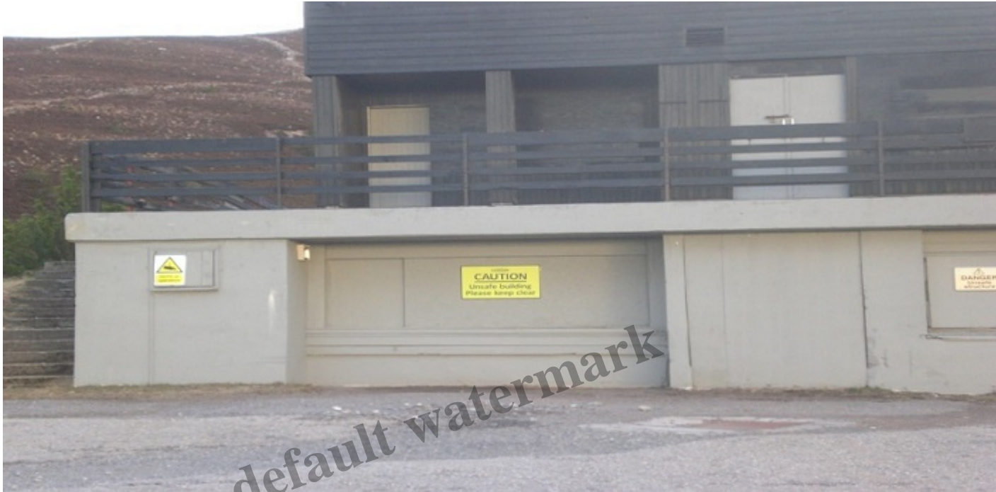
A dilapidated building with signs that say: "Unsafe building, please keep clear"
