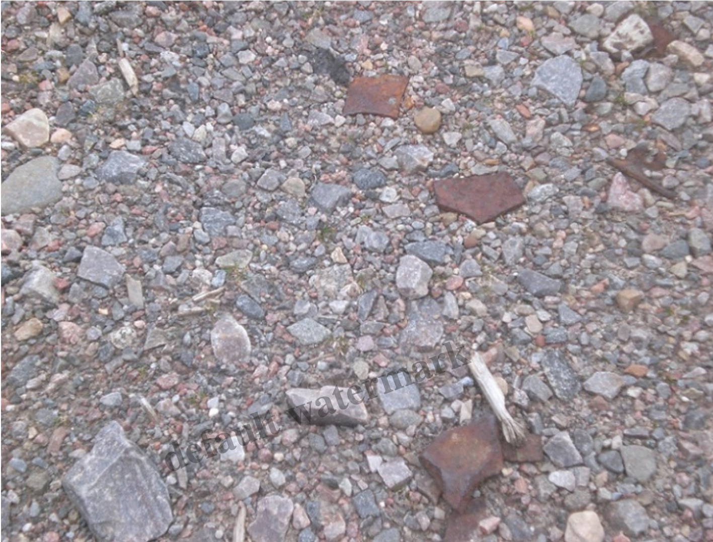
Rusting pieces of metal which are on the ground in the Ciste car park.
