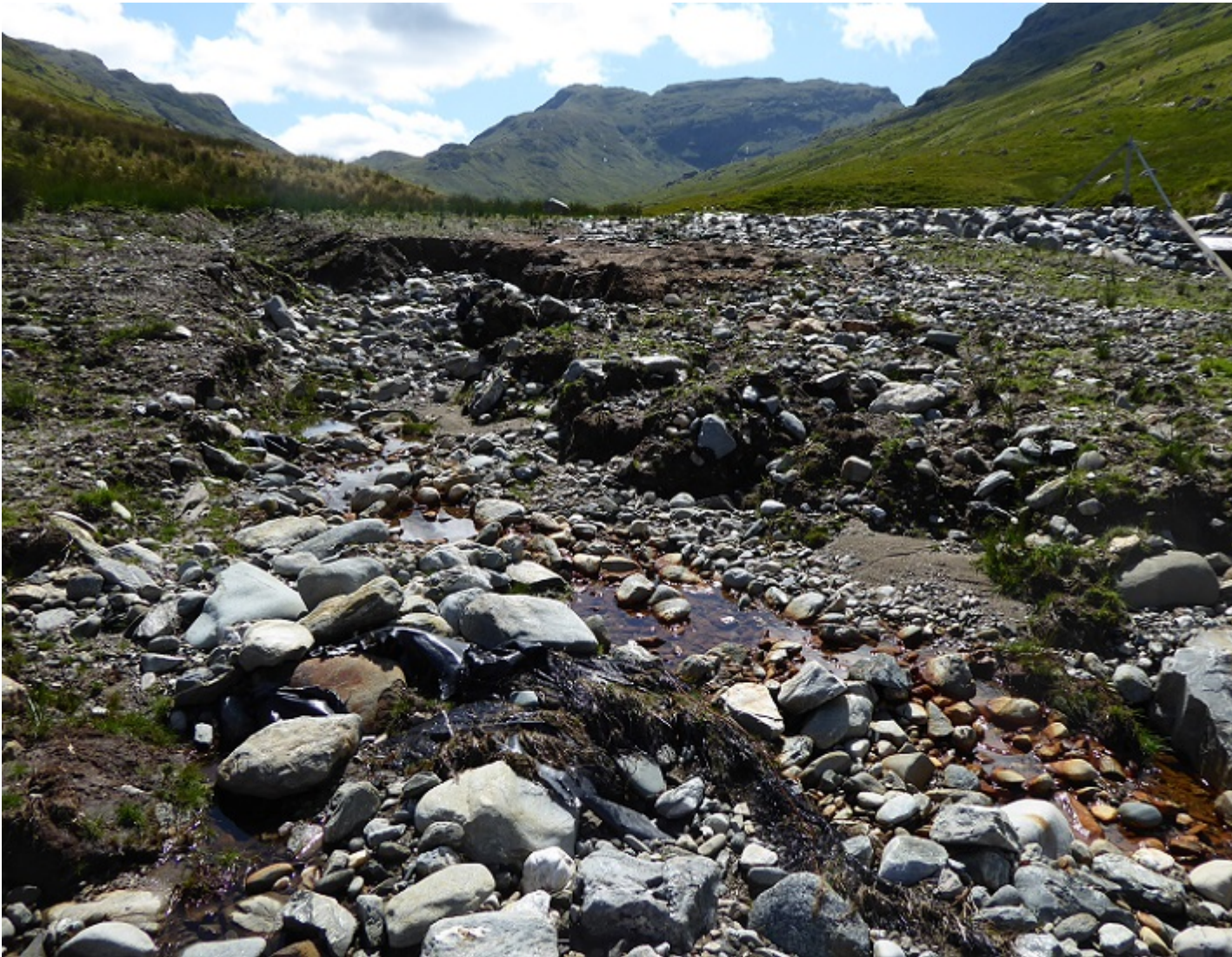
The channel created by the flood has now been “restored” and the peaty area has been separated from the river by the new bank
