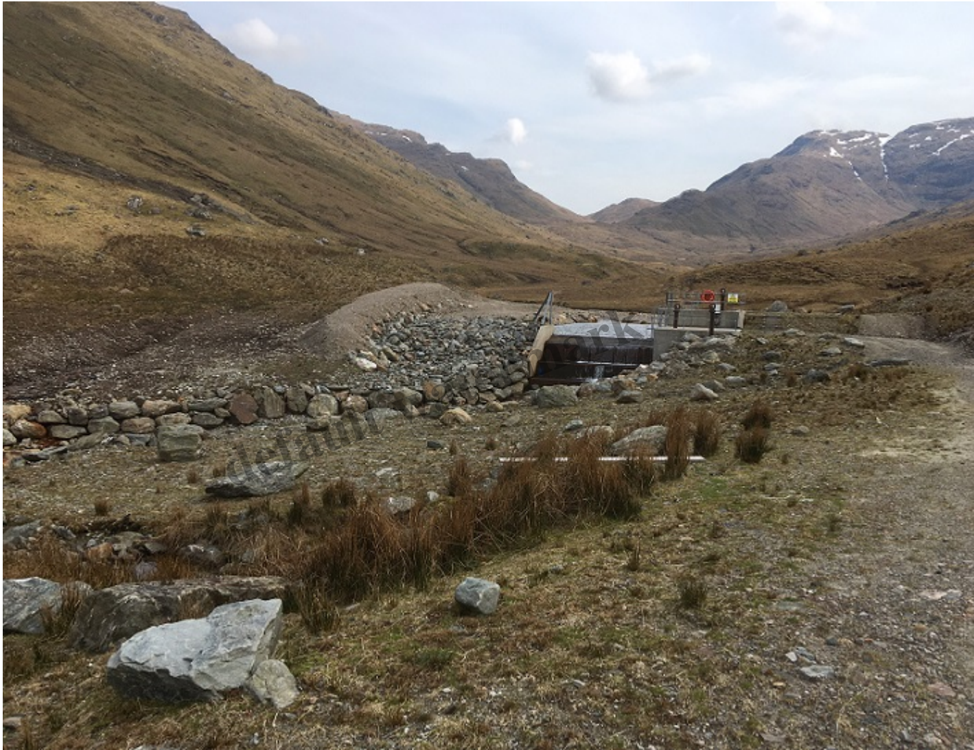
The Upper Glen Falloch hydro intake April 2020, looking in Coire Earb with the popular Munro, Beinn a Chroin on the right. Note the new bank, between the area of peat on the left and the boulderly slope by the intake. Photo Credit Helen Todd.
