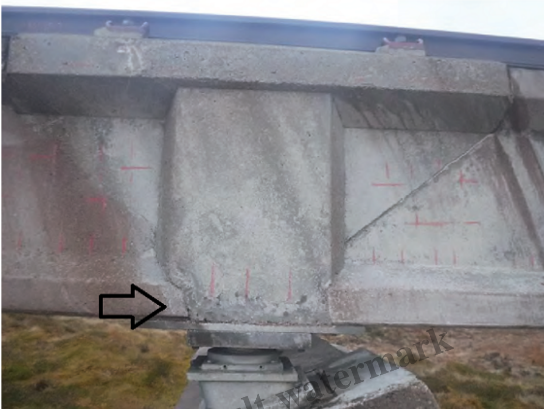
Photo credit COWI report Page 293, plate 38, pier 69, arrow points to possible earlier pour.
