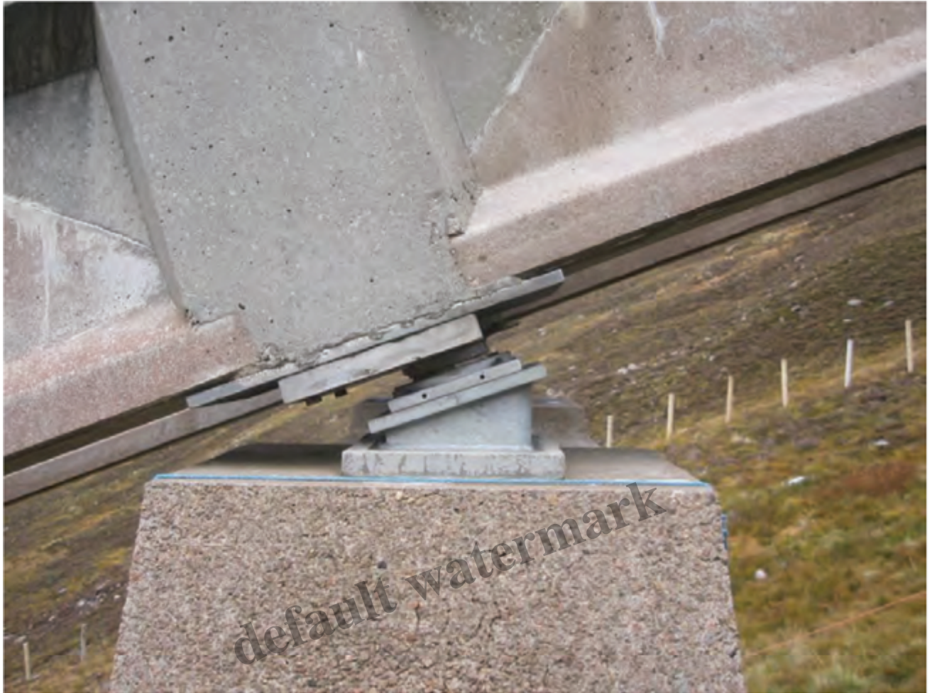
Figure 2-9 Bearing misalignment (refer defect 5)
