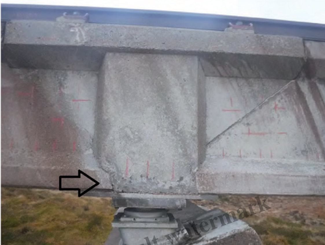
Photo credit COWI report Page 293, plate 38, pier 69, arrow points to possible earlier pour.
