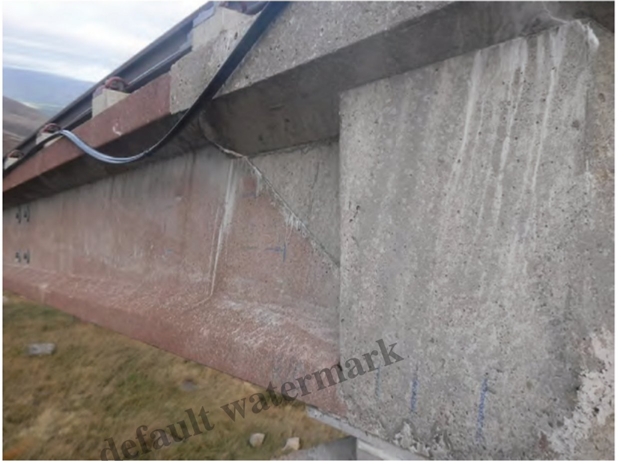
Plate 31 - General view of surface markings to Pier 56 Right Beam down
