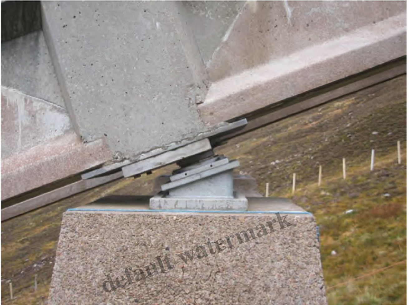
Figure 2-9 Bearing misalignment (refer defect 5)
