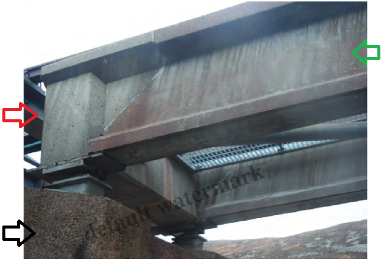
Plate 24 - General view of surface markings to Pier 53 Right Beam, left support up.
