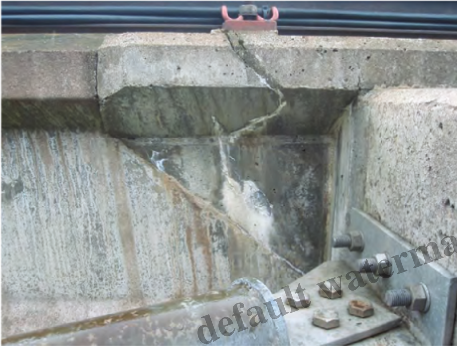
Figure 2-6 Cracking at a pier 9 (refer defect 1)
