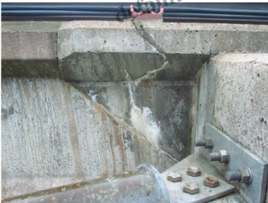
Figure 2-6 Cracking at a pier 9 (refer defect 1)
