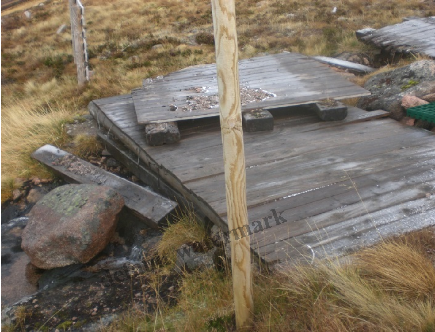
Bridge over the burn that runs down towards the Pump House on the lower Zig Zags known as chicken gully, so called as its less steep than the Cas gunbarrel
