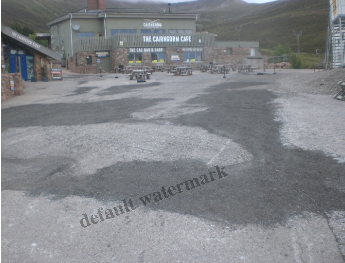
Resurfaced car park – note the loose material
