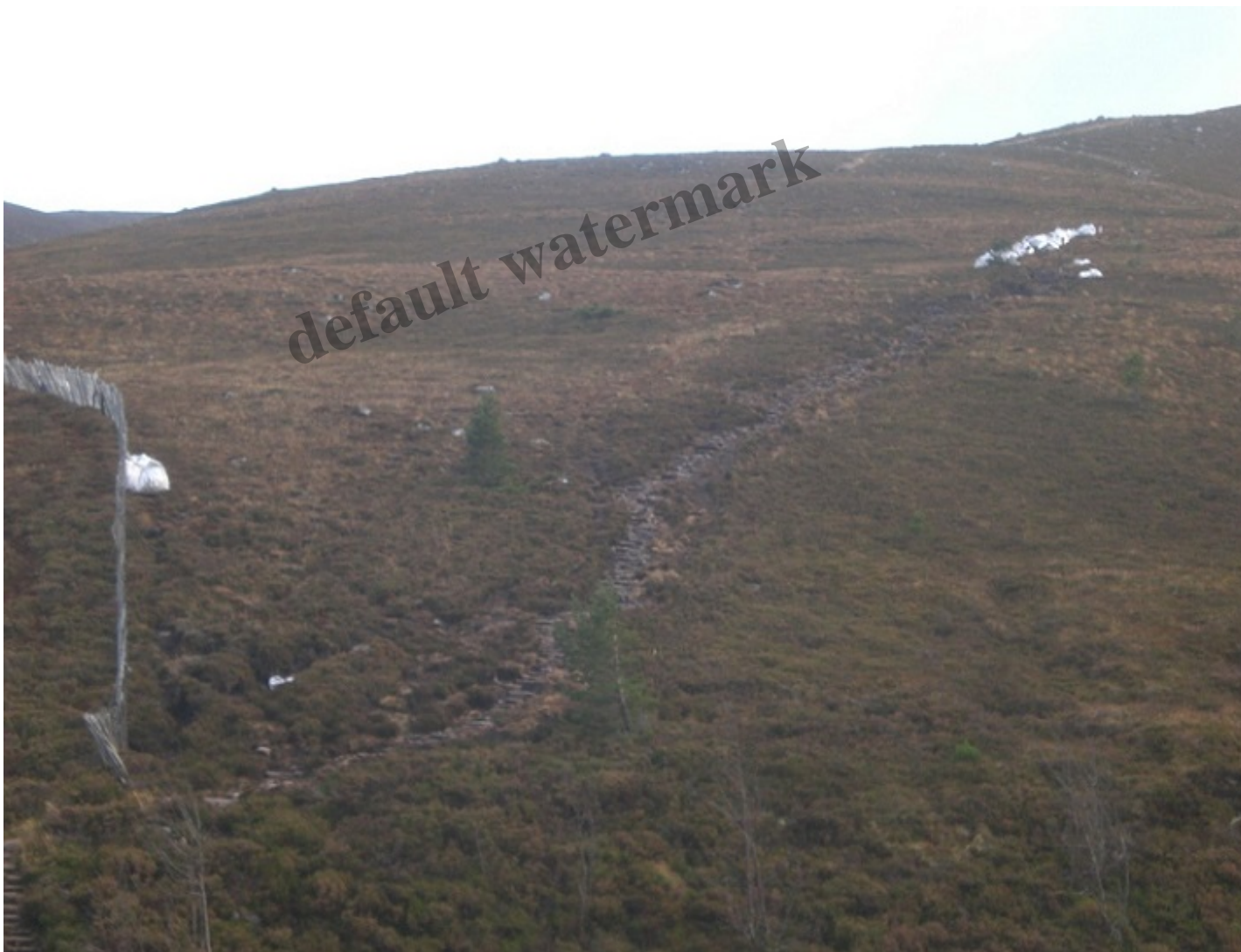
Stone path under construction on the east side of Coire na Ciste
