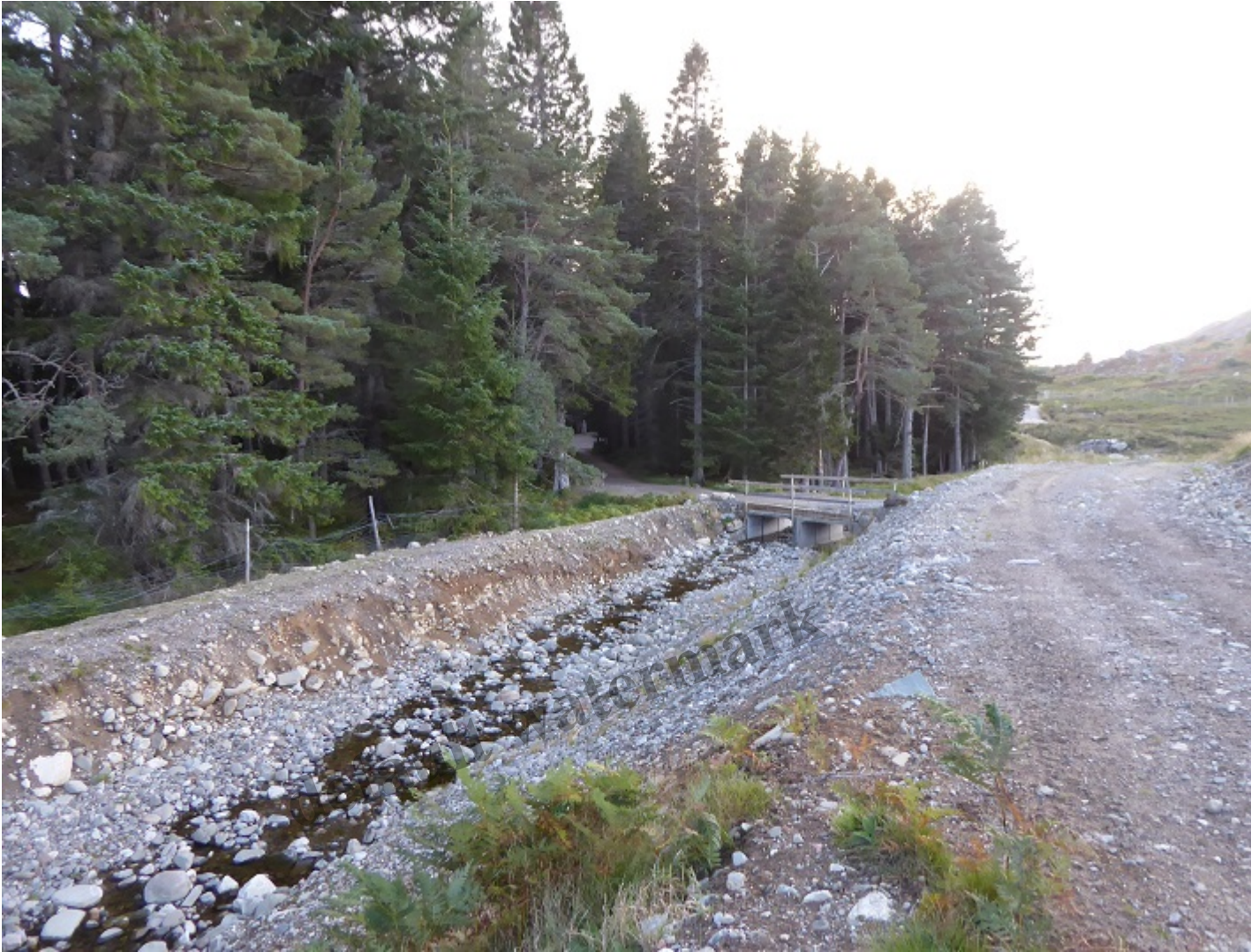
The bridge is taken by the track that takes the West side of the Allt Mor to Carn an Fhreicheadain
