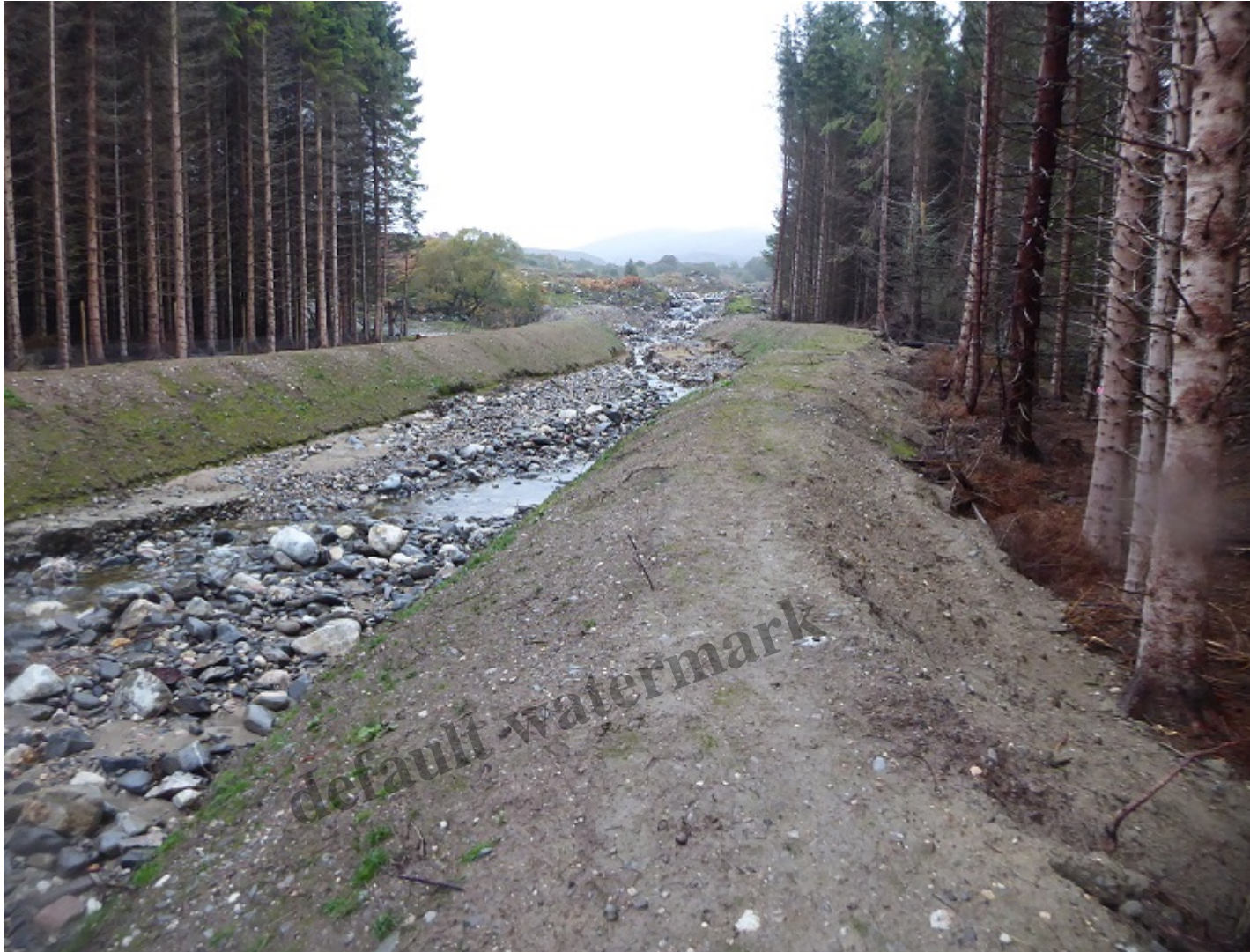
October 2018. The nearest photo I have for how the earth banks looked after construction
