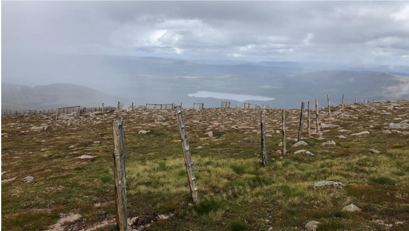
Ruined fencing on the Bynack piste from the M2 into the Aonach Bowl. Photo credit Alan Bratley Autumn 2020
