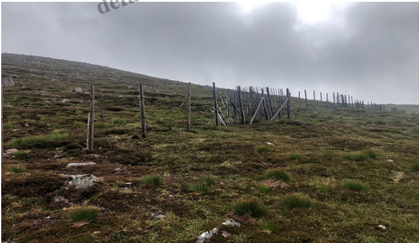
More dilapidated fencing a bit further up the East Ciste. Photo credit Alan Bratney Autumn 2020
