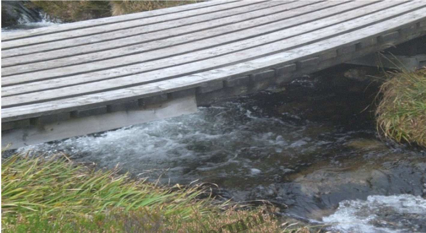
The bridge over the Allt na Ciste which leads to the East Ciste 'path'. Photo credit Alan Bratley Autumn 2020
