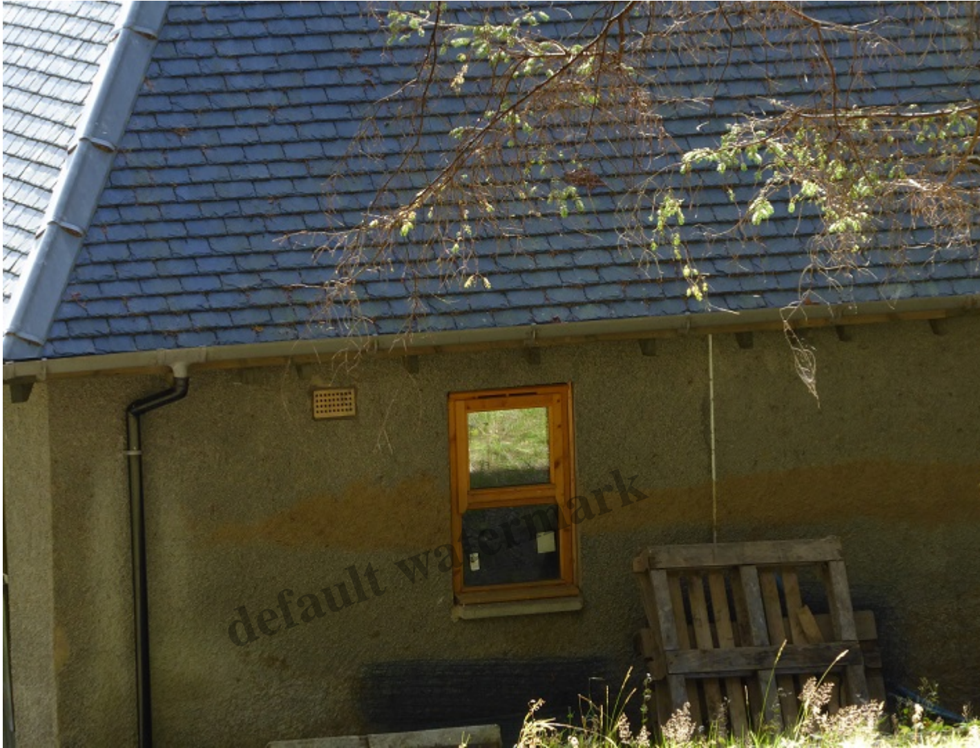
The brown line marks the height of the debris which piled up against a lower building
