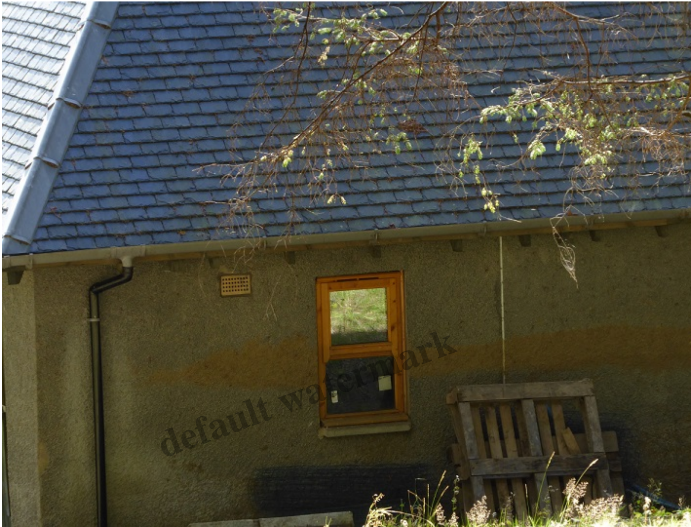
The brown line marks the height of the debris which piled up against a lower building
