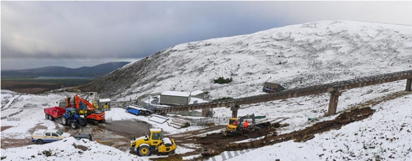
View of the repair works from above the mid-station, with compound on left and pillars 51,52 and 53 visible
