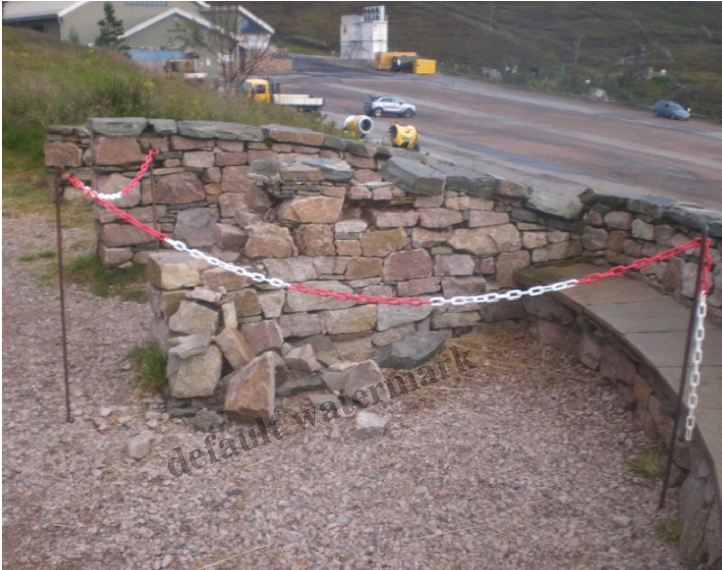
The dangerous section: taken down and roped off [no hazard signage though]
