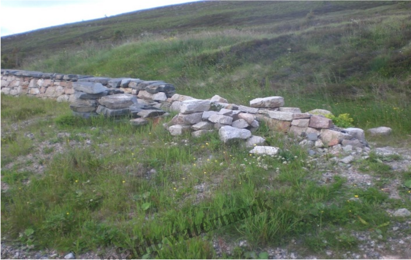
Collapsed stonework. Picture sent to HIE
