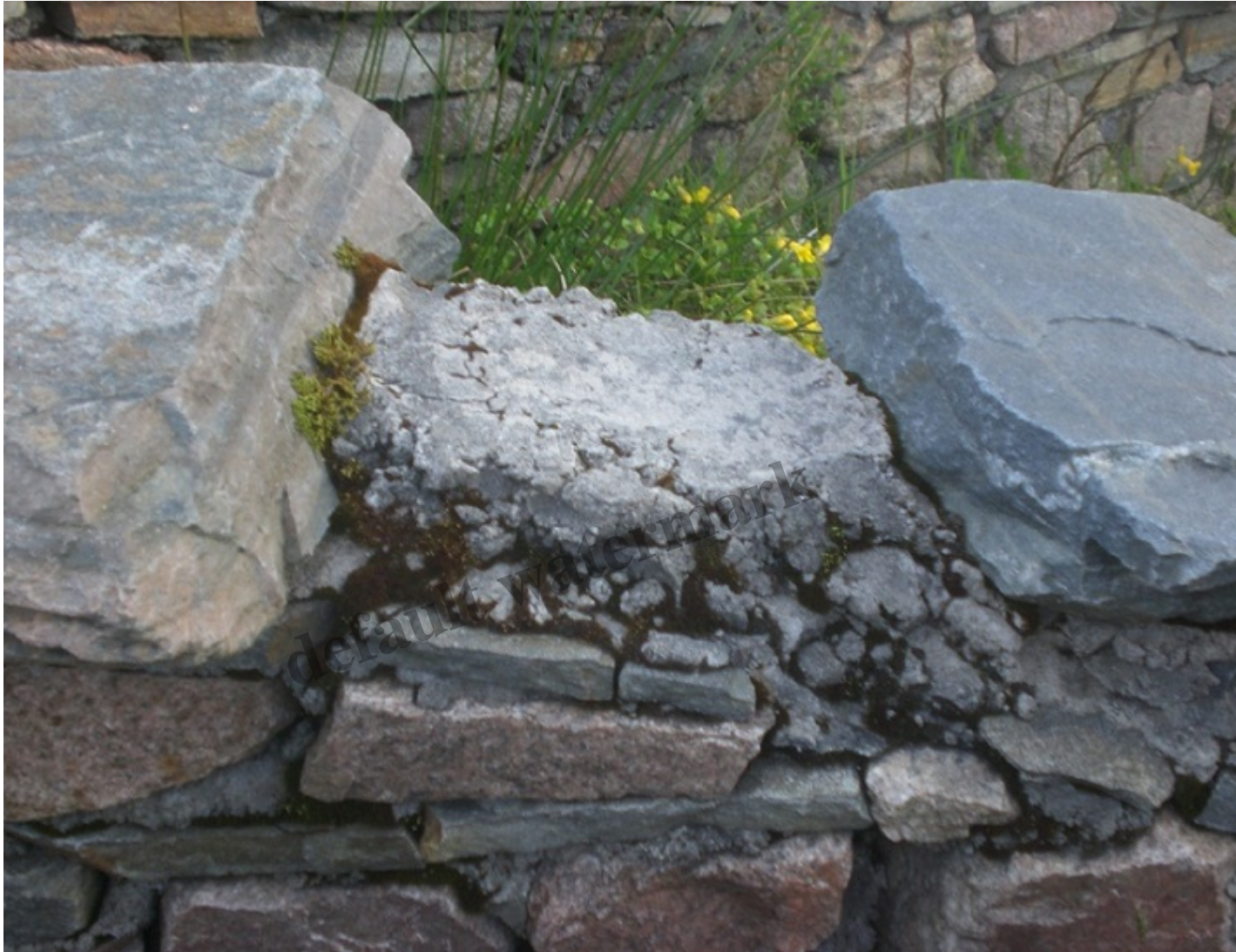
Picture of a missing Cap Stone.....sent to HIE
