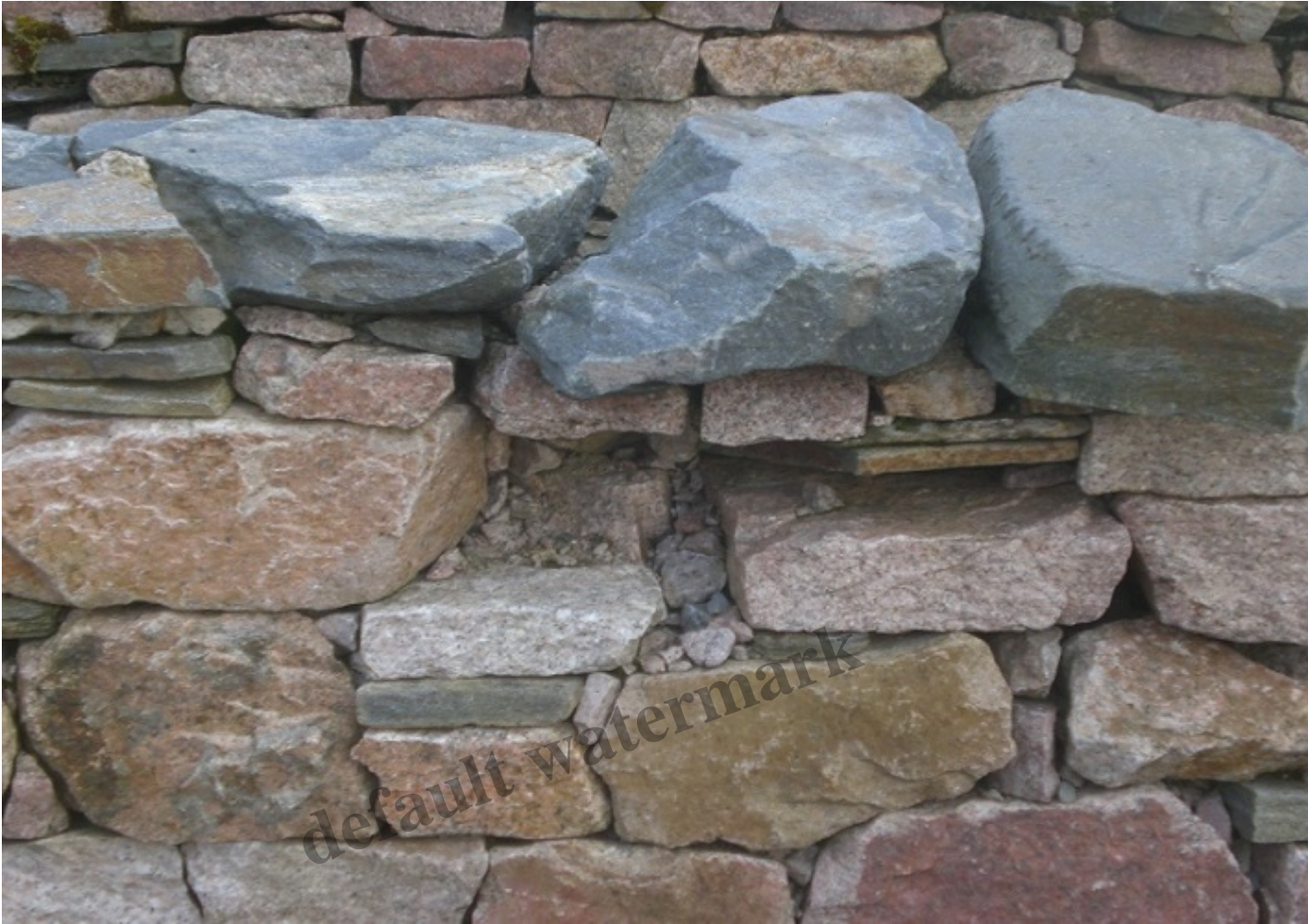
Picture of the missing stone which could have led that section of wall to collapse under the weight of child.....sent to HIE
