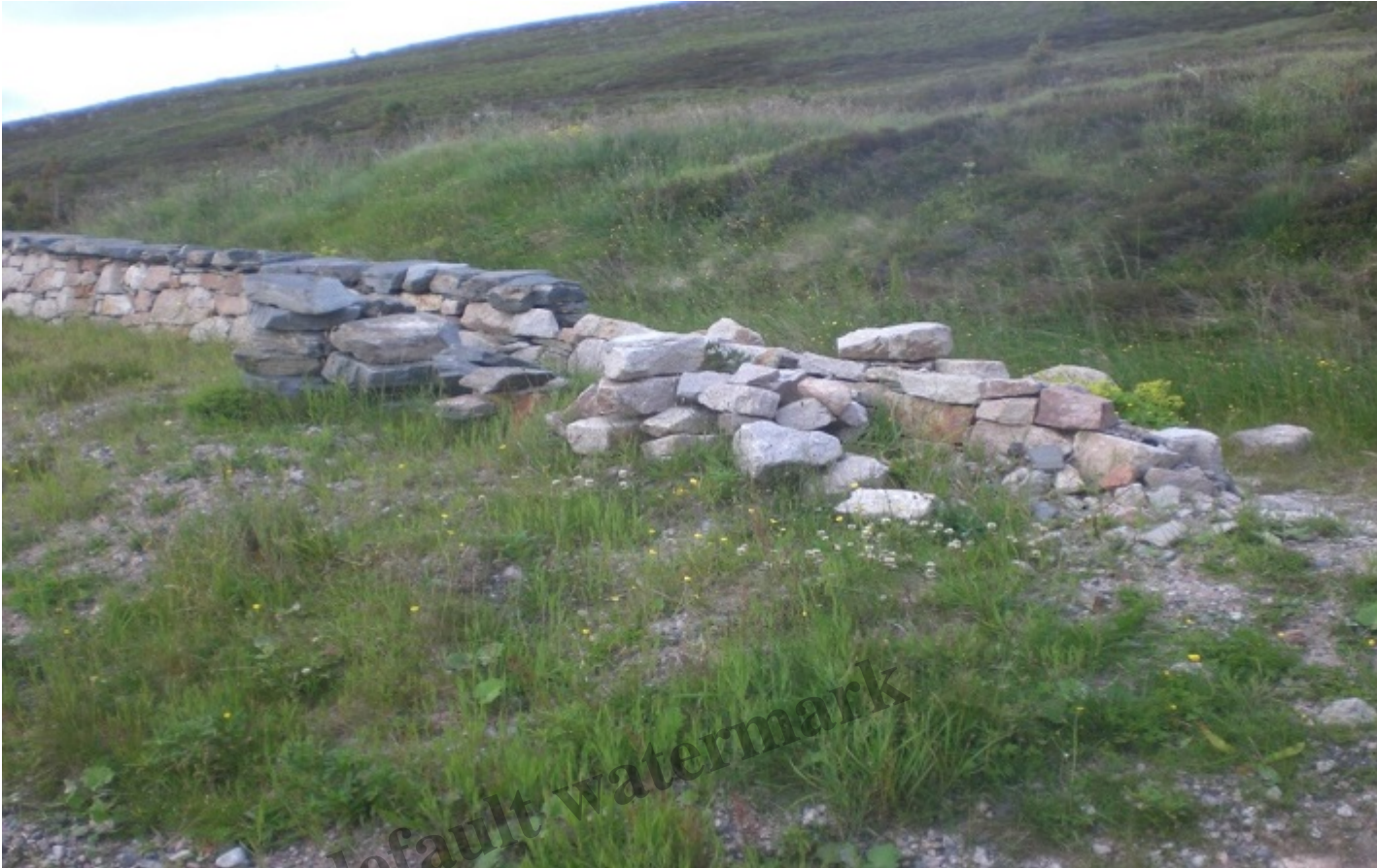
Collapsed stonework. Picture sent to HIE
