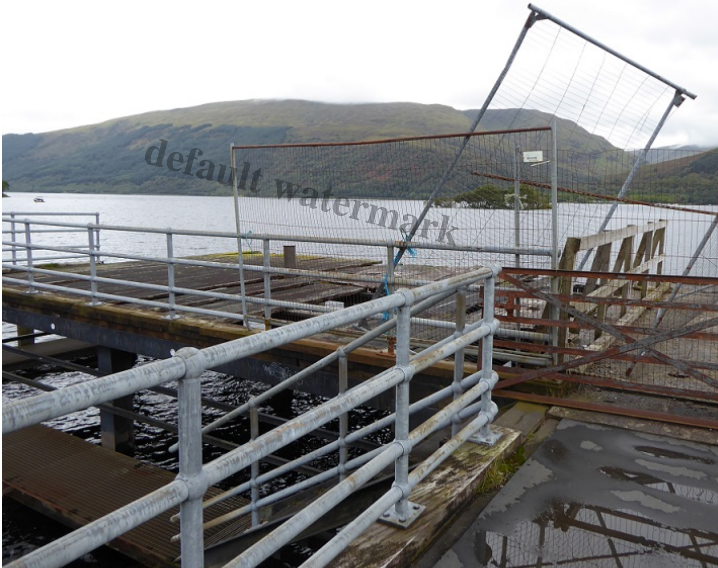
Crumbling visitor infrastructure – Rowardennan pier 16th September
