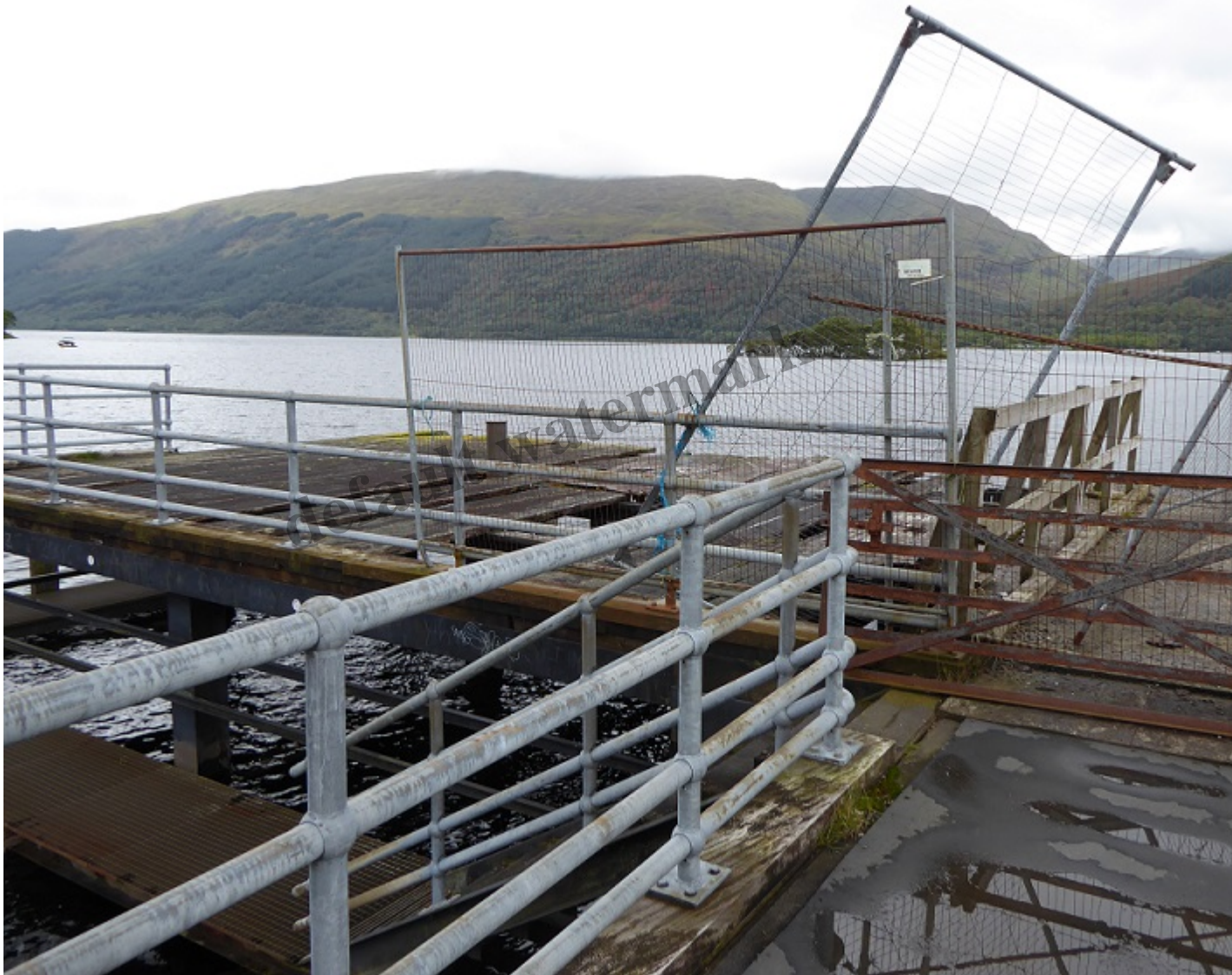
Crumbling visitor infrastructure – Rowardennan pier 16th September
