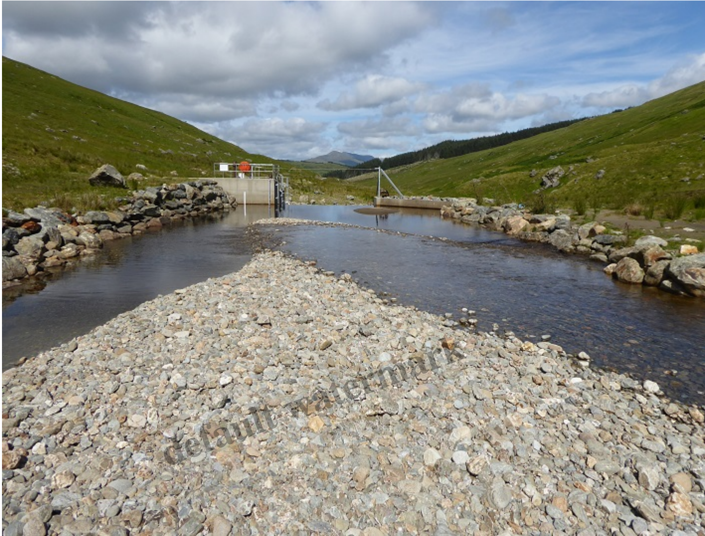
Infilling intake pool August 2020. As the river re-wilds, the hydro is at continuous risk of redundancy
