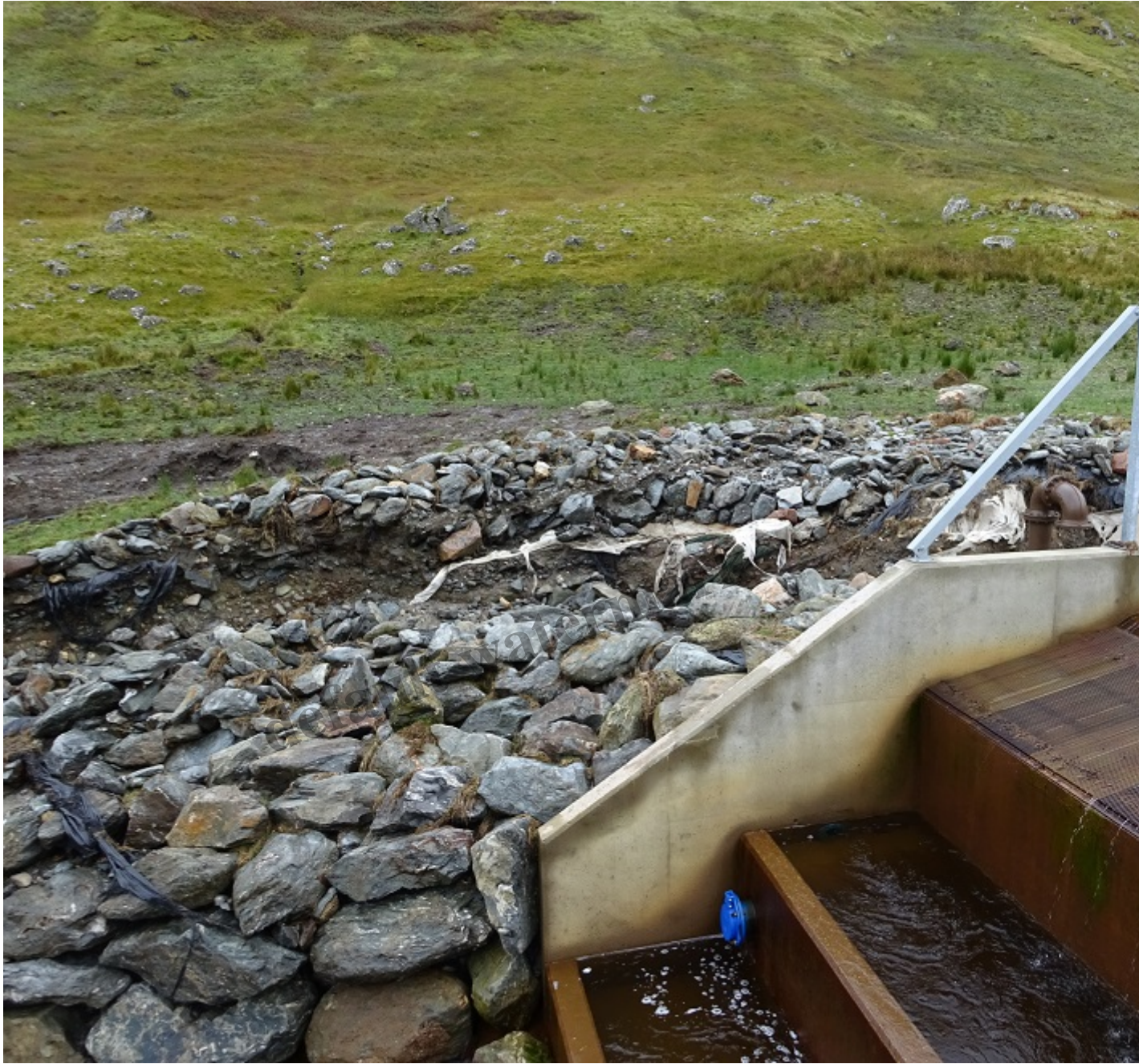
New channel created by overflowing river in August 2019
