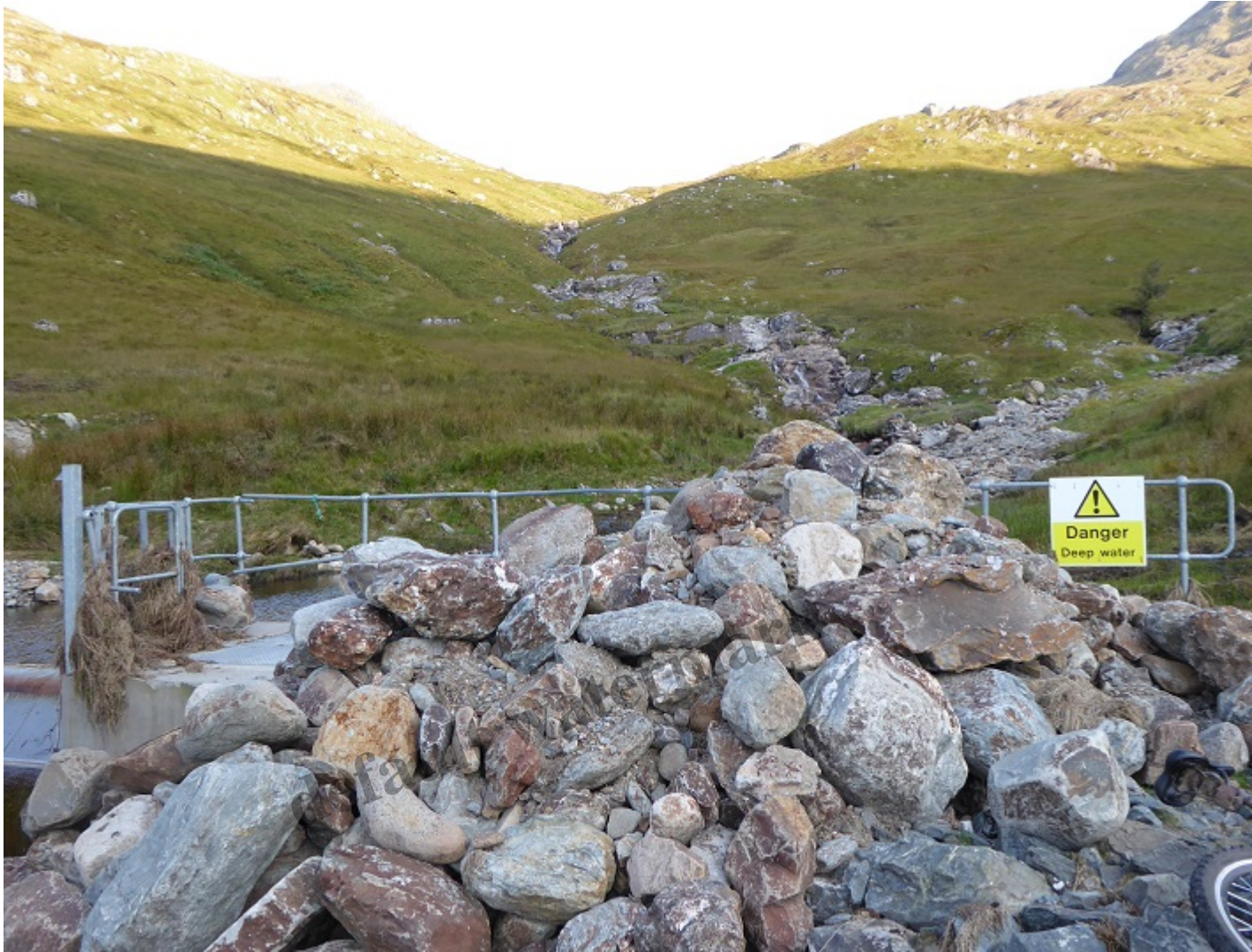
September 2019. A pile of boulders that appeared to have been excavated from the intake pool.
