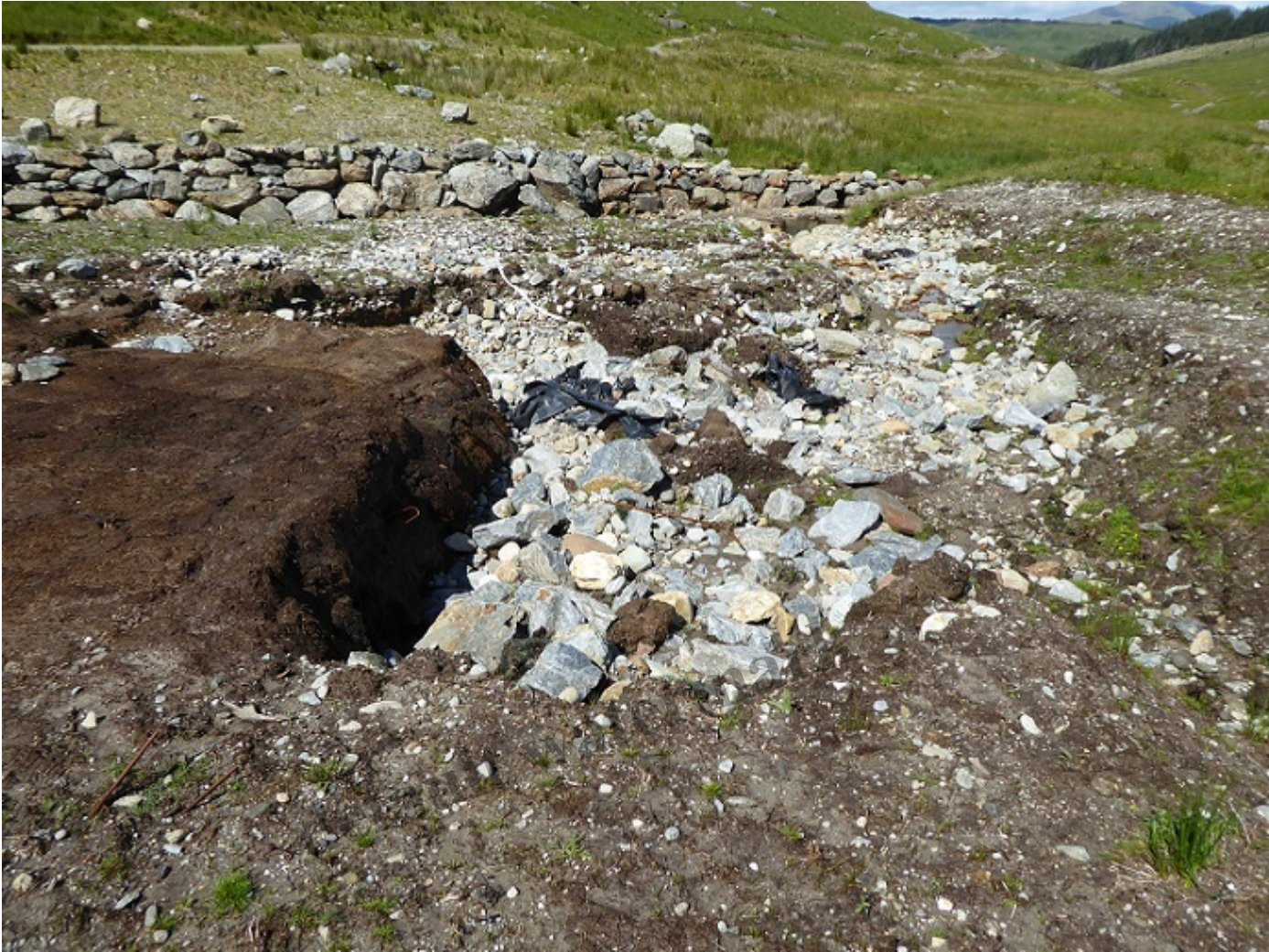
Looking down one of the new channels created by the flood over to far bank of the River Falloch below the intake. A large area of “restored” peat just waiting to be swept away.
