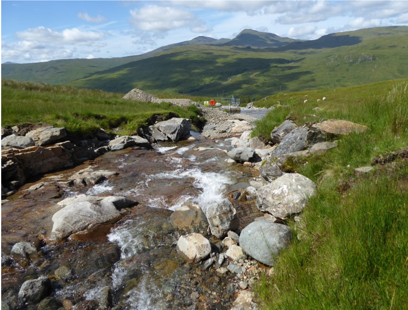
Allt Andoran intake with Ben Oss behind – the flat bit to right of highest part of heap has been created by diggers being driven up onto the heap to drop more stones and boulders. August 2020.
