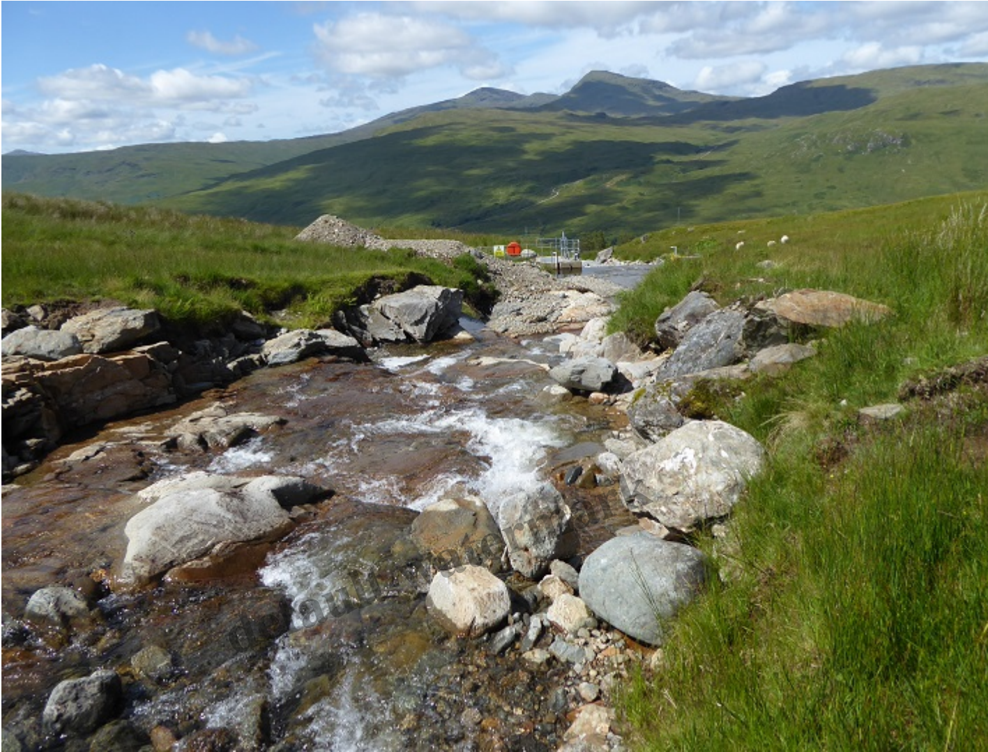
Allt Andoran intake with Ben Oss behind – the flat bit to right of highest part of heap has been created by diggers being driven up onto the heap to drop more stones and boulders.Â August 2020.
