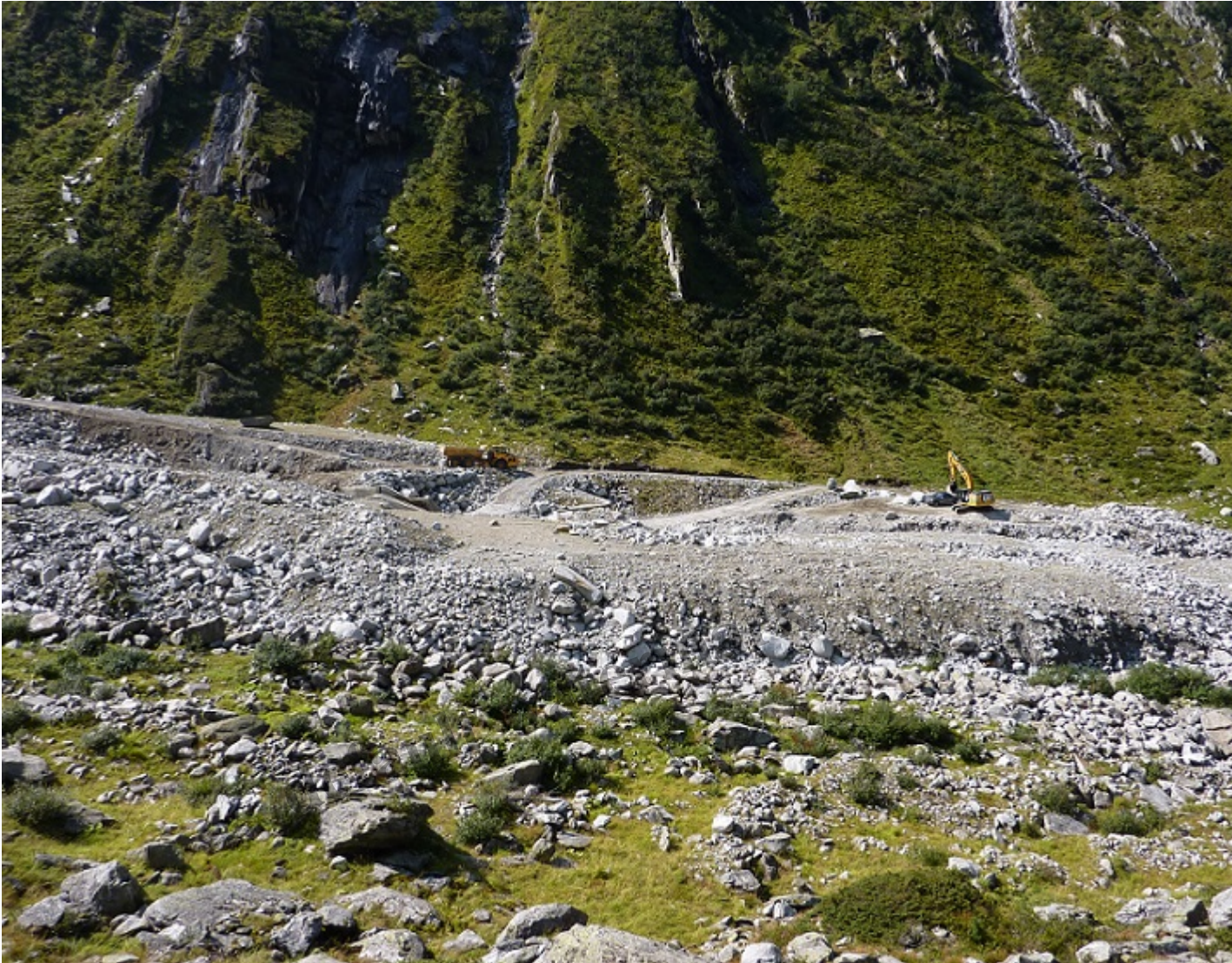
An example from an Austrian National Park – the concrete hydro intake is visible just to the left and forward from the dumper truck
