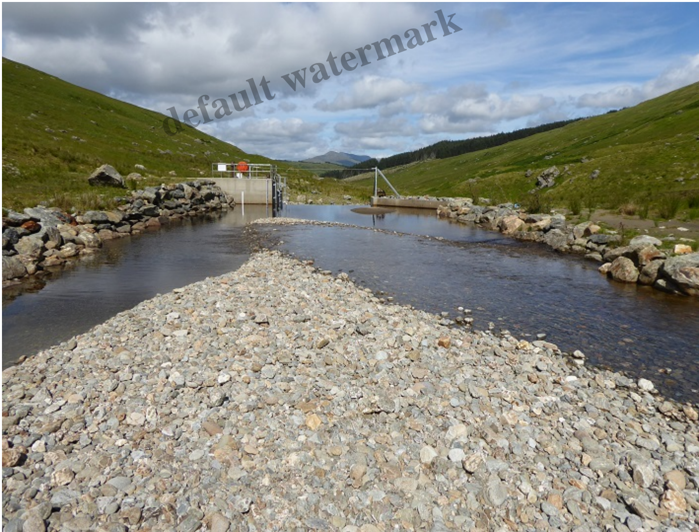
Infilling intake pool August 2020. As the river re-wilds, the hydro is at continuous risk of
