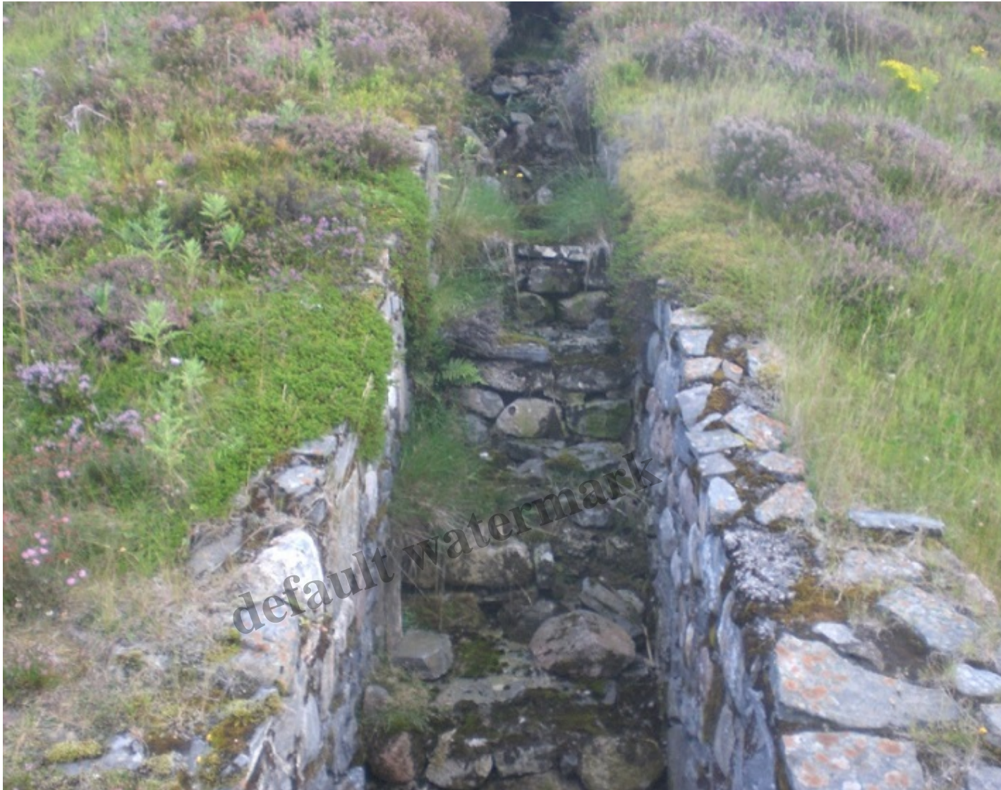
Link Road drainage channel. Unmaintained and as a result starting to fall to pieces.
