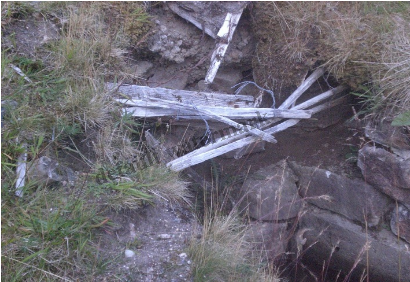
Lower Cas Car park. A drainage channel coming down from the upper car park.
