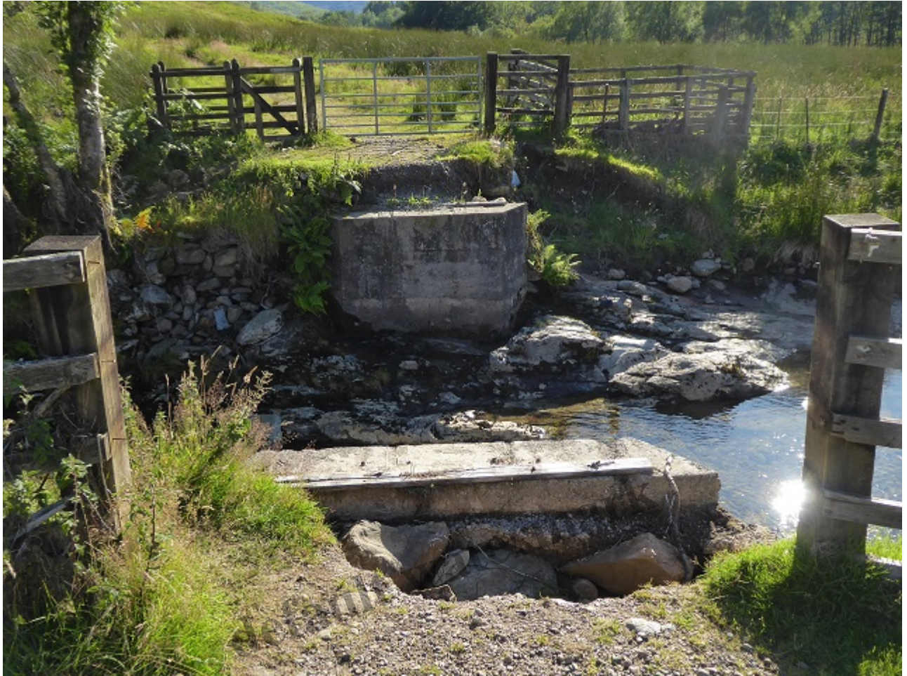
Looking back down Glen Falloch. Note the material eroded out from behind the pillar
