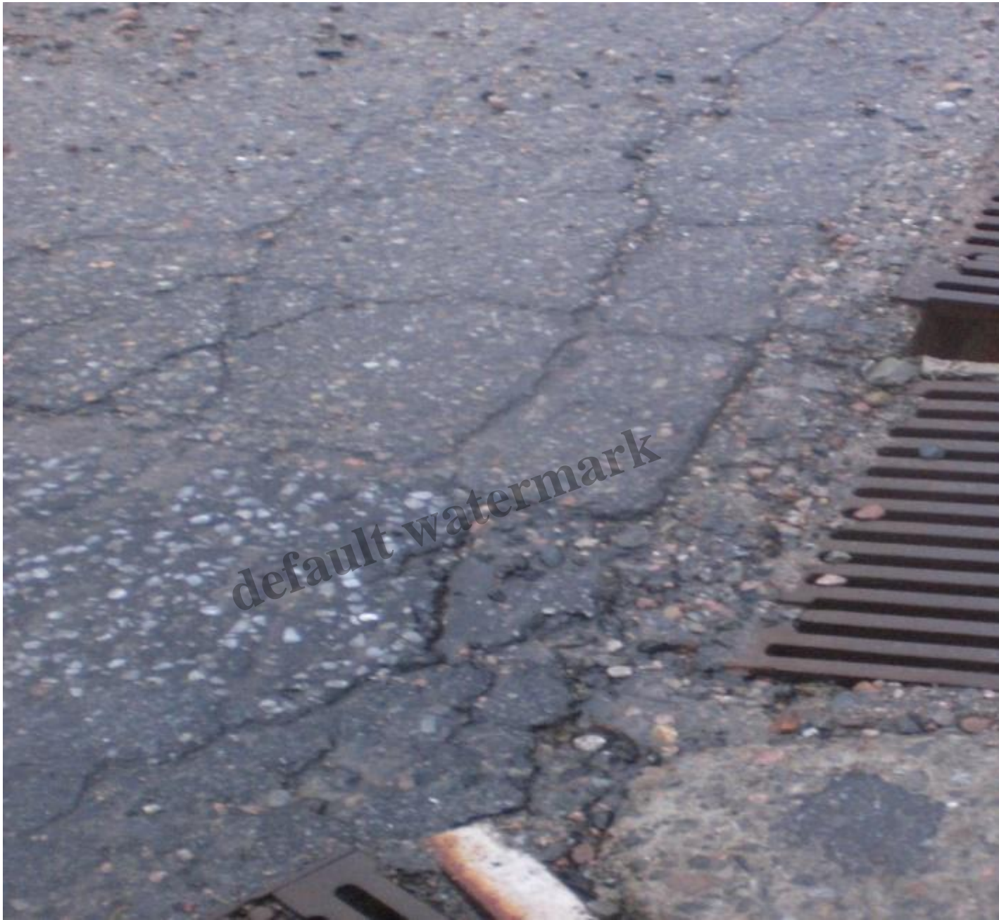
Damaged metal drain cover in November 2019.
