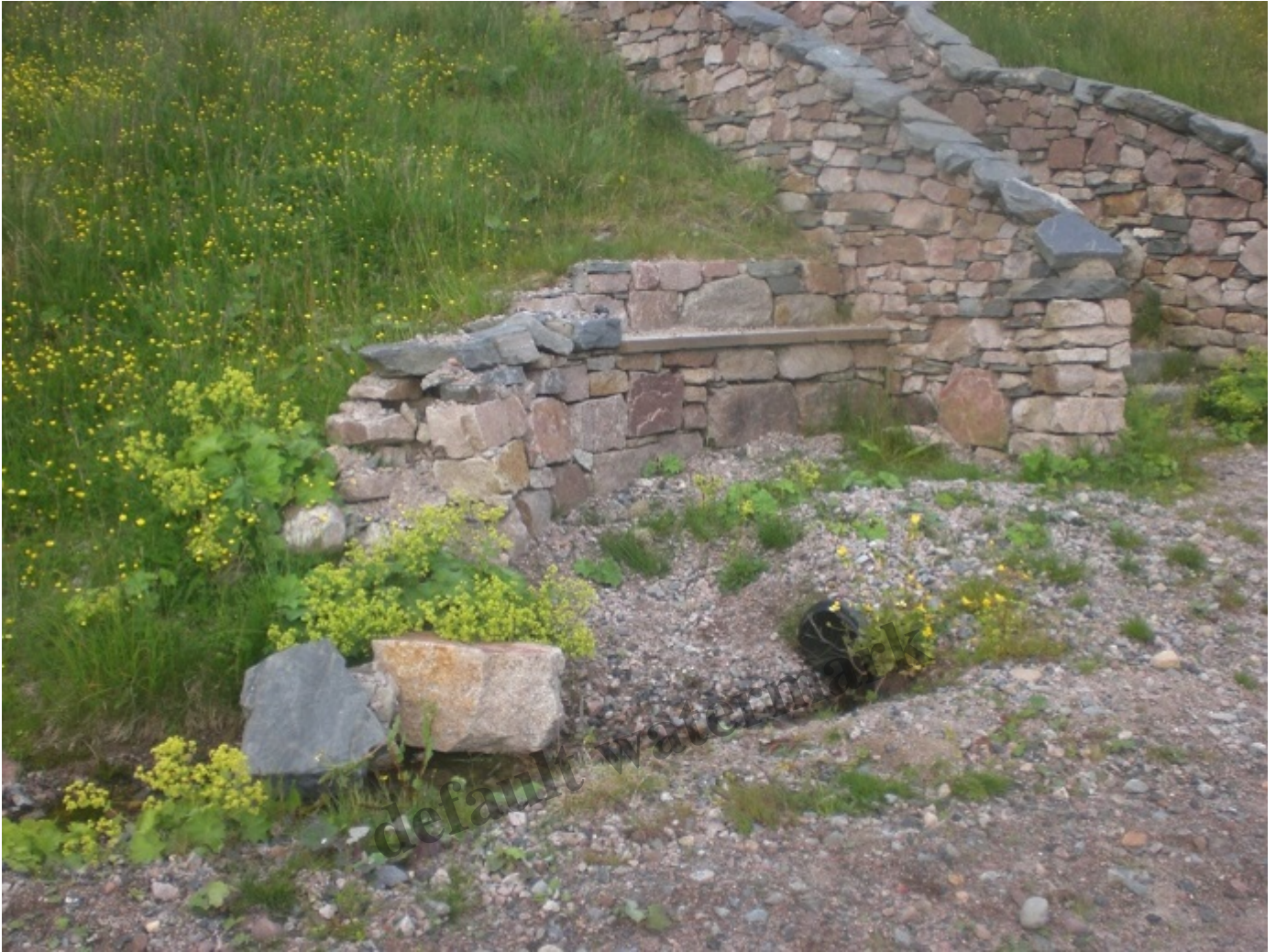
Collapsed dyking adjacent to the stairway.
