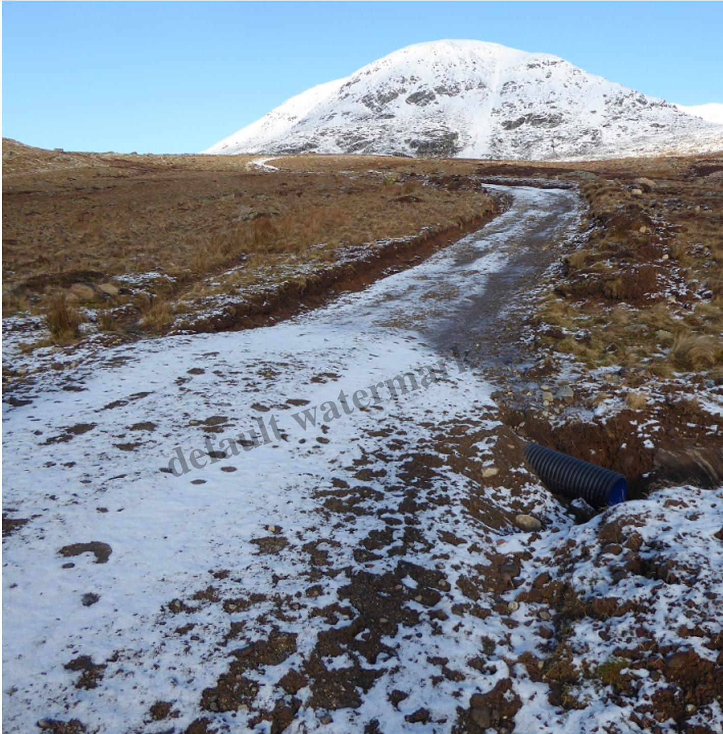
Part of the upper section of the Glen Clova hotel hill road that must now be removed
