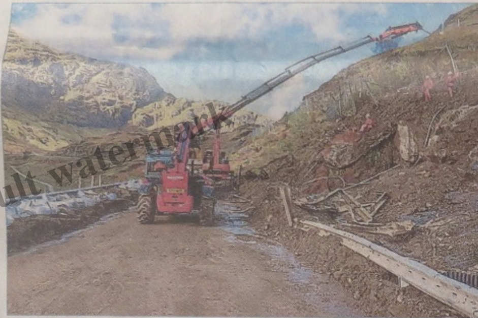
The Rest and Be Thankful is notoriously prone to landslips
