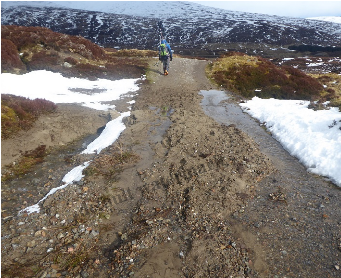
Eroded silt and other material washed down to below the steeper section. Note the depth of silt to the ditch
