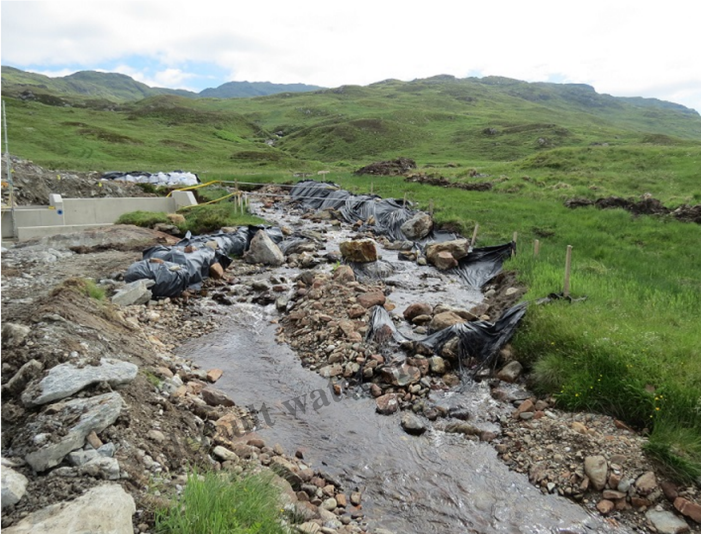
Diversion channel dug through peatland to construct hydro intake 2016. Note the piles of turf and peat to the right.
