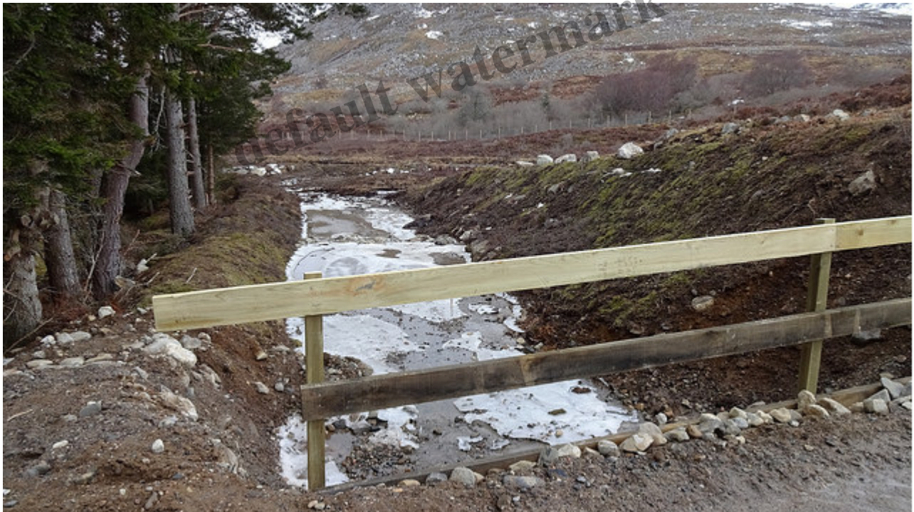
In April 2018 Highland Council published this view of the overflow from the road bridge near the intake
