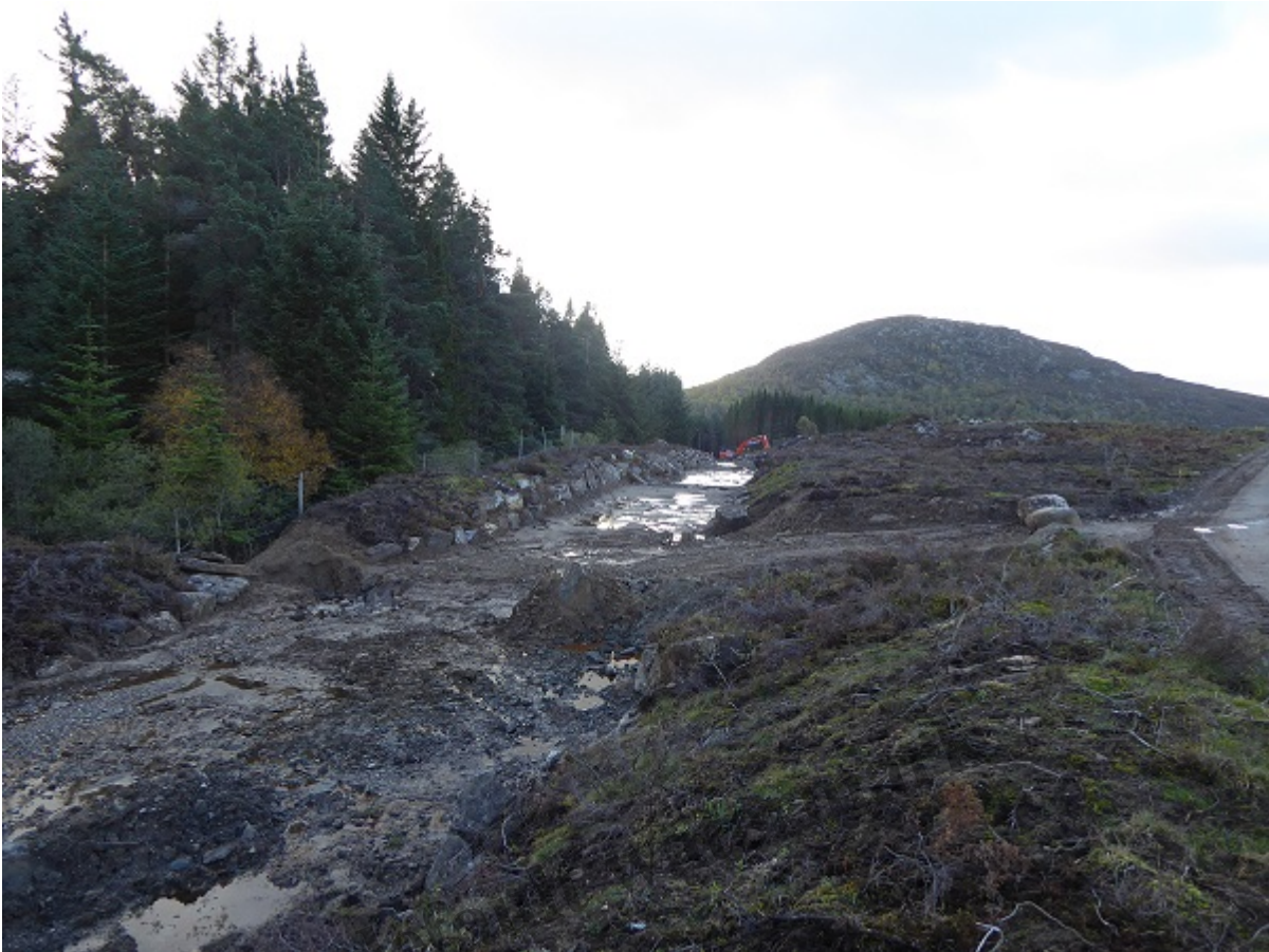
The overflow channel under construction October 2017 – note the new bank on the left
