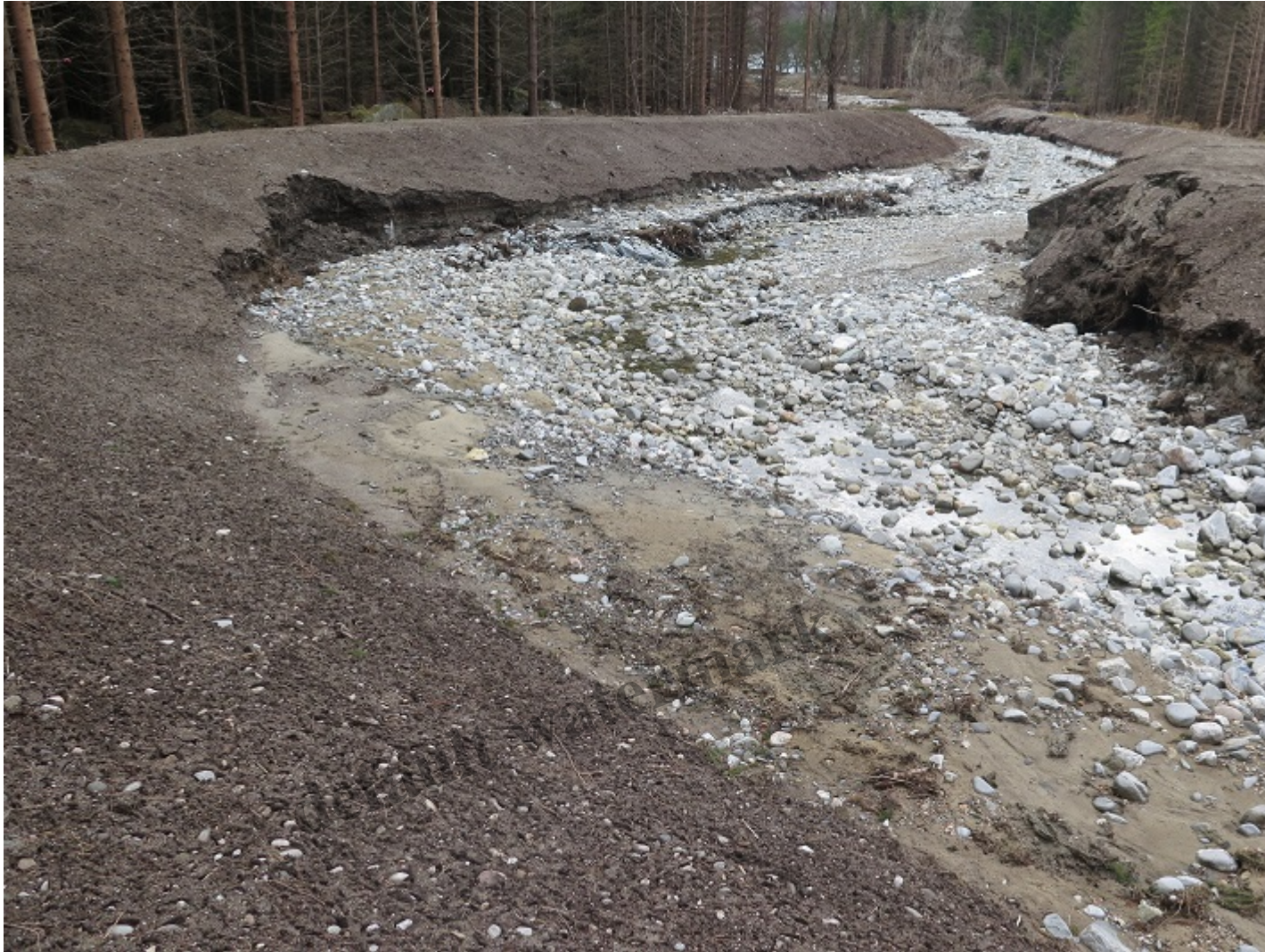
Channel with manicured banks already eroding – 29th April 2018. This view was not shown by High
