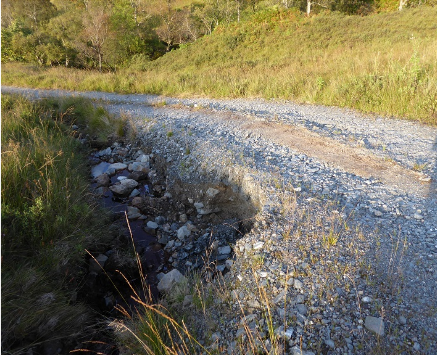
Edge of track eroded away by flood and now threatened with collapse
