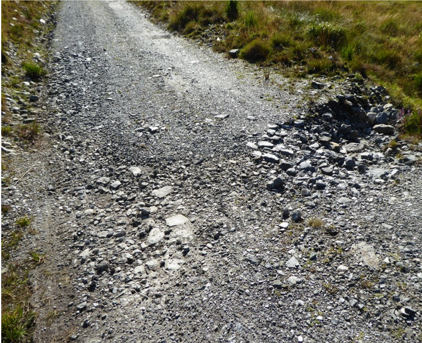
Collapsed section of road caused in part by water flowing across it and eroding its edge.
