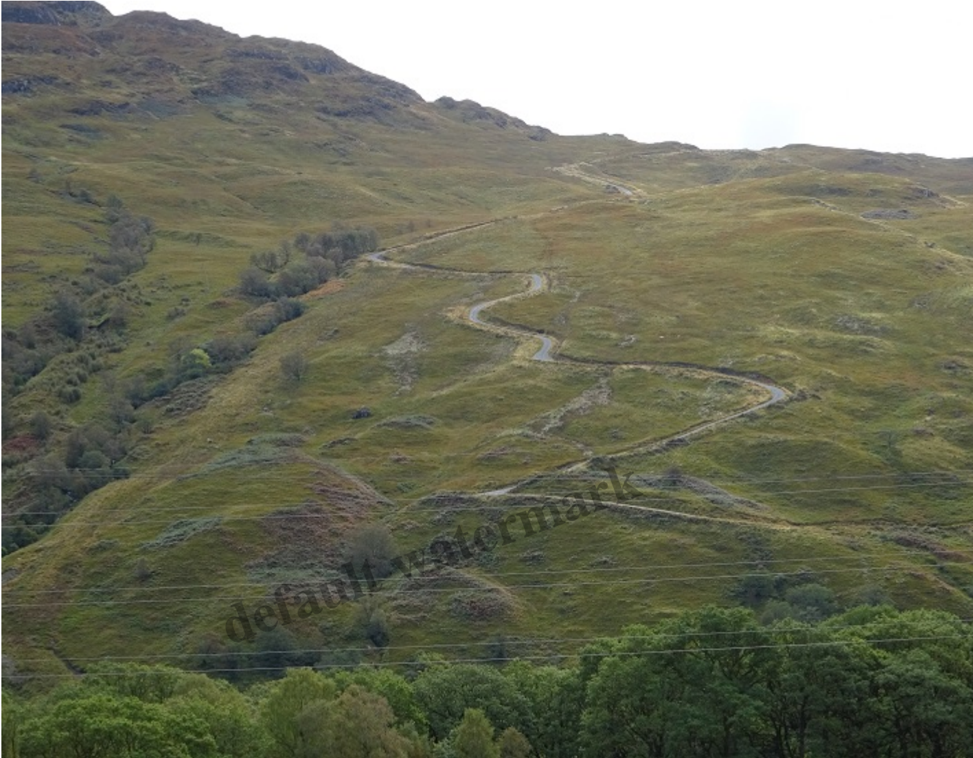
Ben Glas hydro road showing how material has been swept down from the road – from the second bend – onto the slopes below. Photo Credit Kevin McGrath Sept 2019
