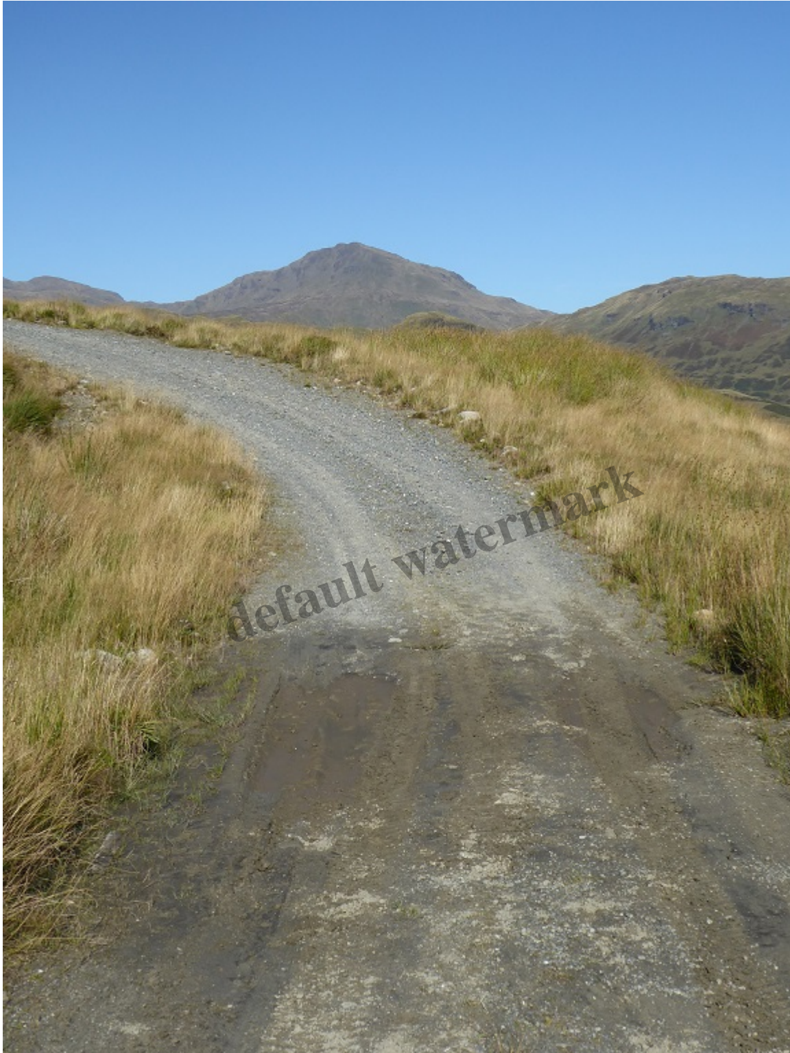
Silt, washed out from the road, accumulating in a dip
