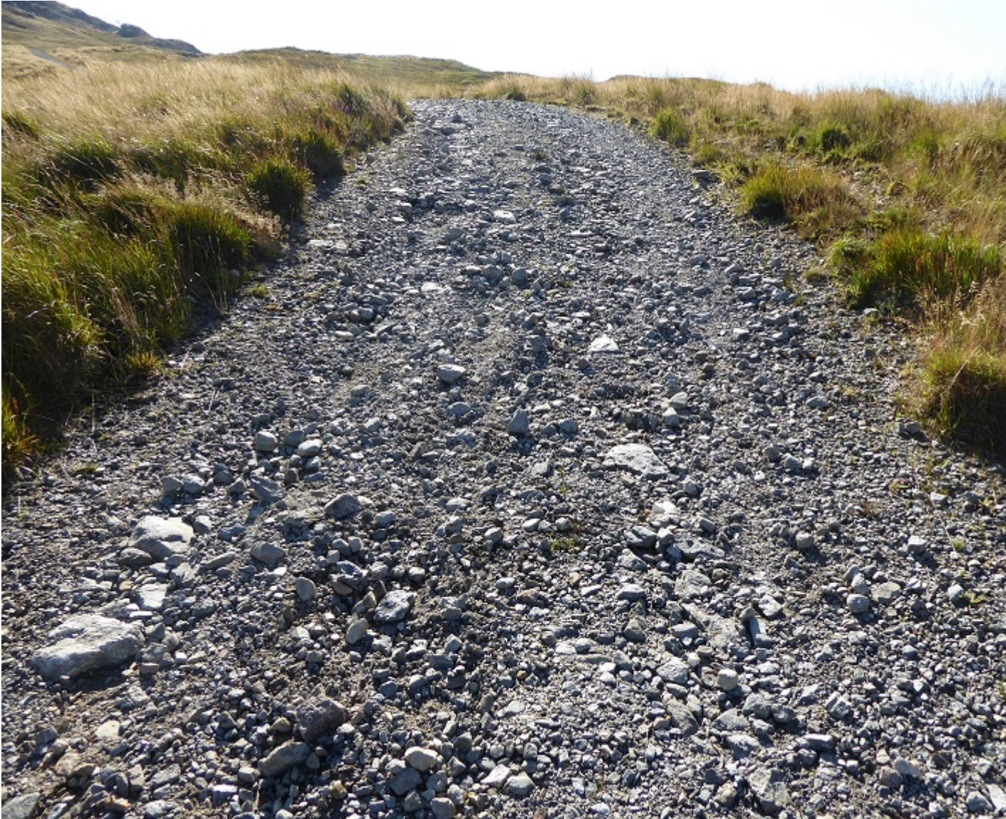
Example of section of road where the fine material has been washed out and where larger stones have started to be moved by the water.
