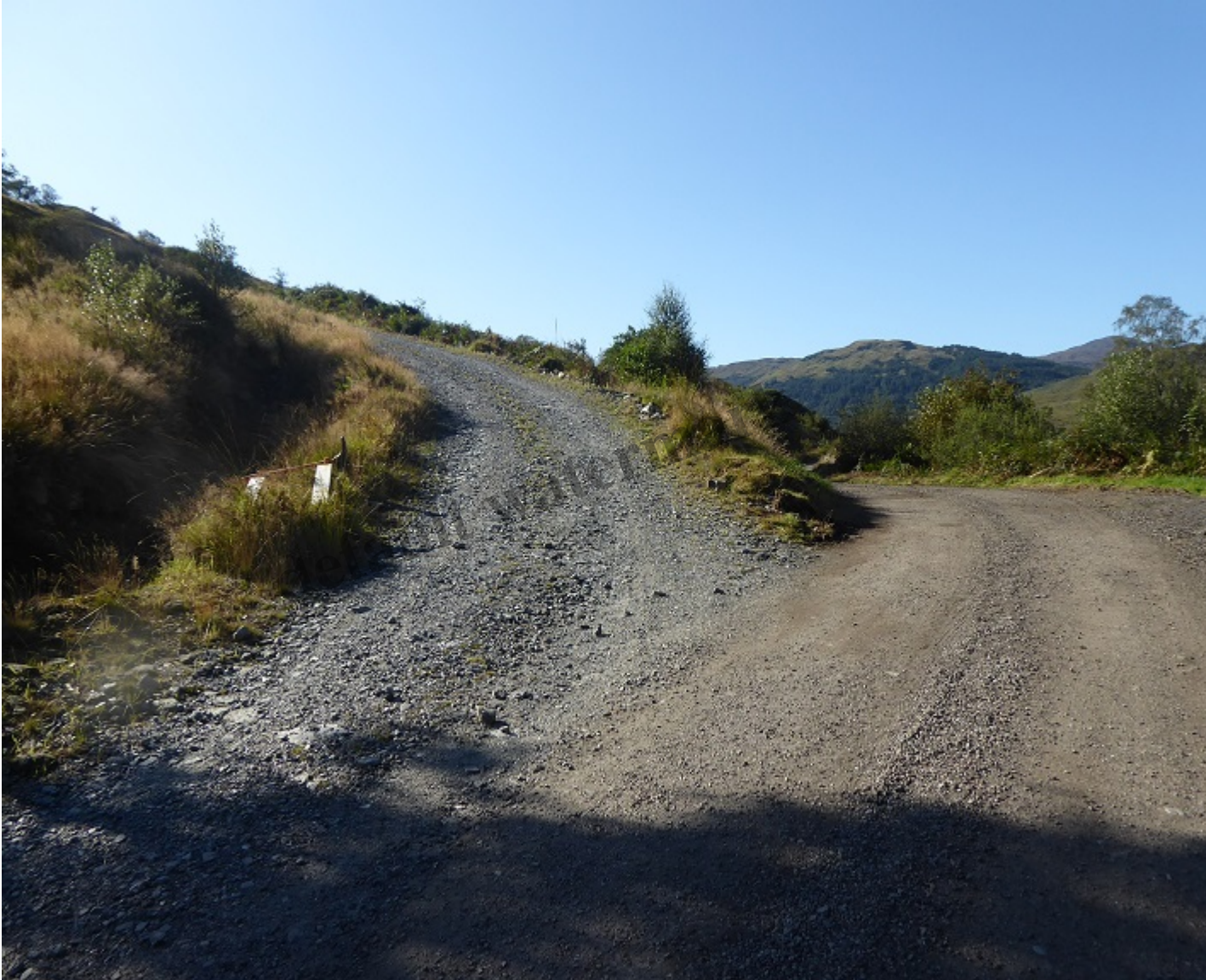
The start of the new Ben Glas hydro hill road illustrating the contrast between its surface, which is already eroding significantly, and the surface of the road below which has retained much finer material
