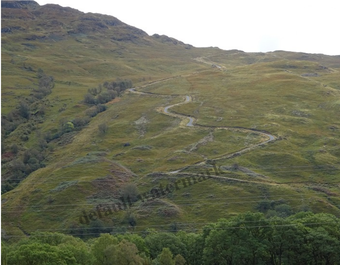
Ben Glas hydro road showing how material has been swept down from the road – from the second bend – onto the slopes below. Photo Credit Kevin McGrath Sept 2019
