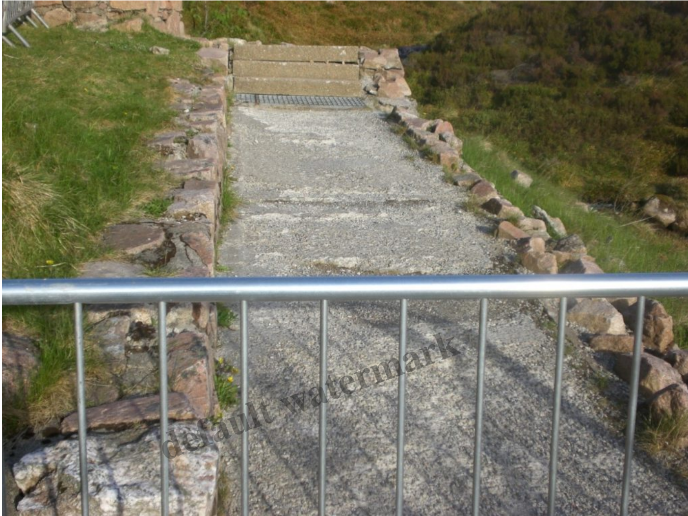
Access around the Daylodge has been closed for months due to the unsafe condition of the path and steps
