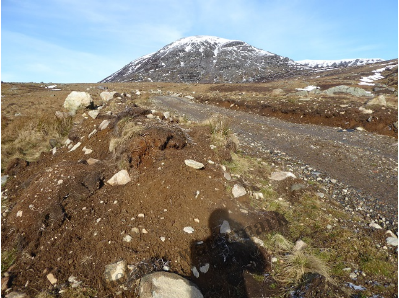
Is this the start of the section of the road which the CNPA has decided is “new”? There is clear evidence that the road has been excavated out of the hillside (bank of earth on left). Feb 2019.
