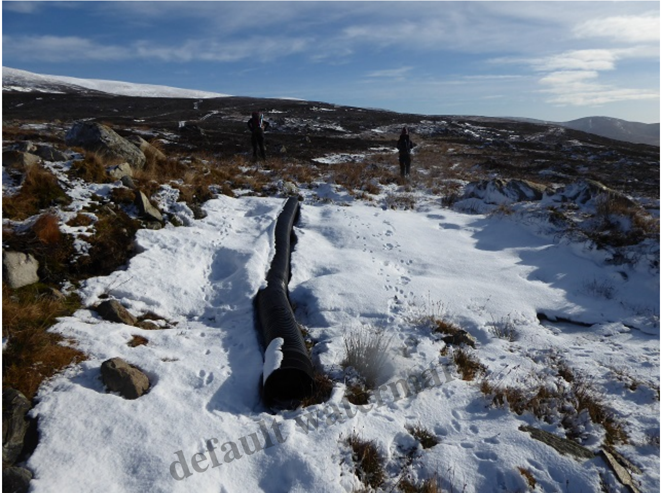
Drainage pipe laid down beyond “end” of constructed road by very boggy section of ATV track leading to hydro intake
