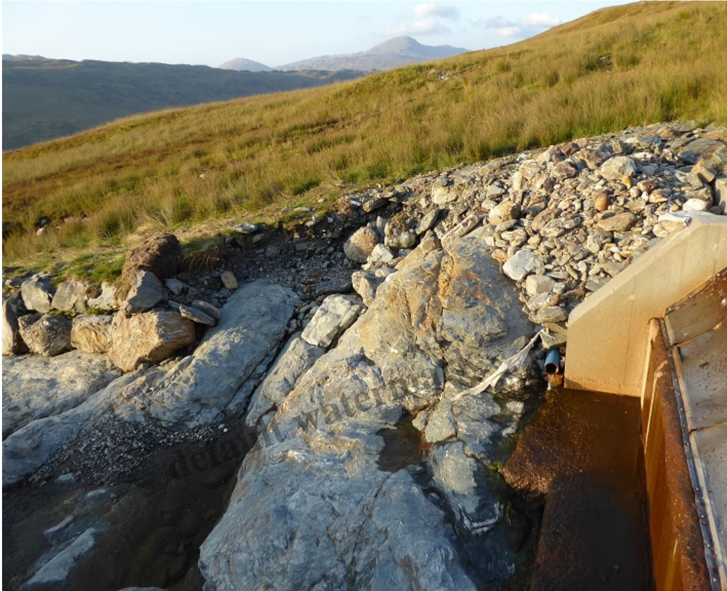
Large chunk of restored bank removed from below Allt Andoran Intake, leaving bare bank behind – E Chalum in distance. Both banks below this intake have been seriously damaged. Photo Author.
