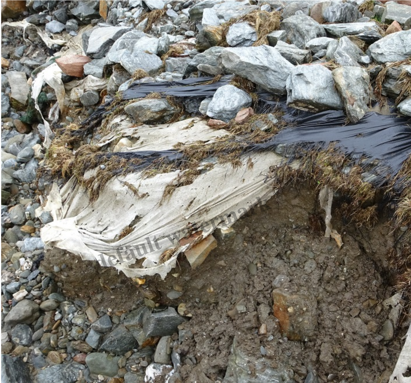
Eroded bank and ripped up sheeting below the Upper Falloch intake. Photo Credit Kevin McGrath
