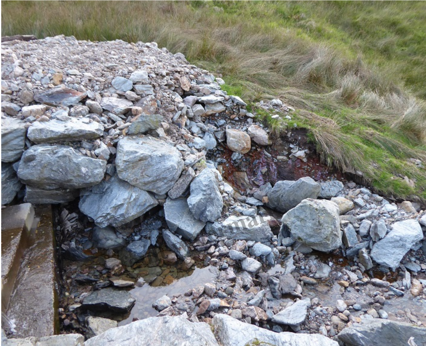
Damaged bank below the second of the Allt a Chuillin intakes
