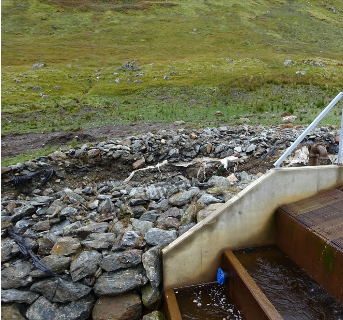
The artificial embankment at the Upper Falloch intake used to reach the top of the concrete walls and away from between them to the new bank opposite. Photo credit Kevin McGrath
