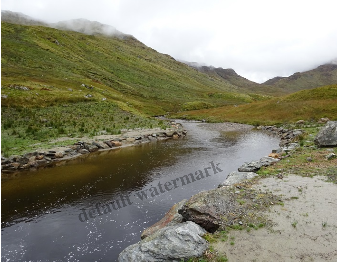
Looking across the intake pool to the rip rap bouldering embankment September 2019 – it now looks far more natural than it did four months ago. Photo credit Kevin McGrath.
