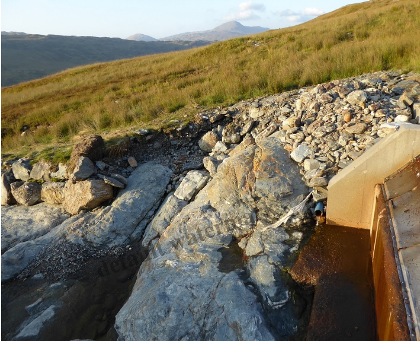
Large chunk of restored bank removed from below Allt Andoran Intake, leaving bare bank behind – E Chalum in distance. Both banks below this intake have been seriously damaged. Photo Author.
