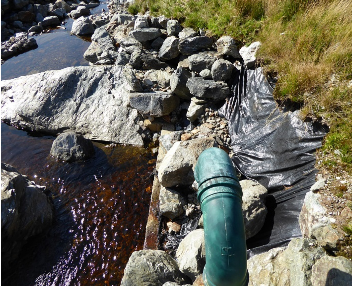
Another example at Ben Glas. The sheeting also stops roots penetrating into the soil below binding
