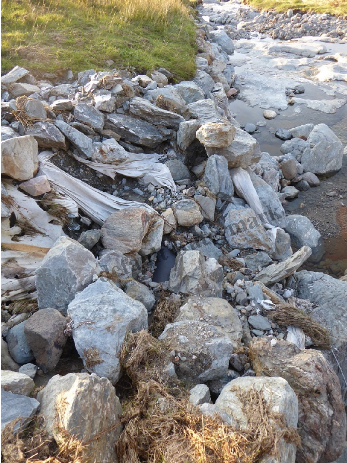
Left bank below Allt Andoran, with cloth sheeting and section of pipe visible centre
