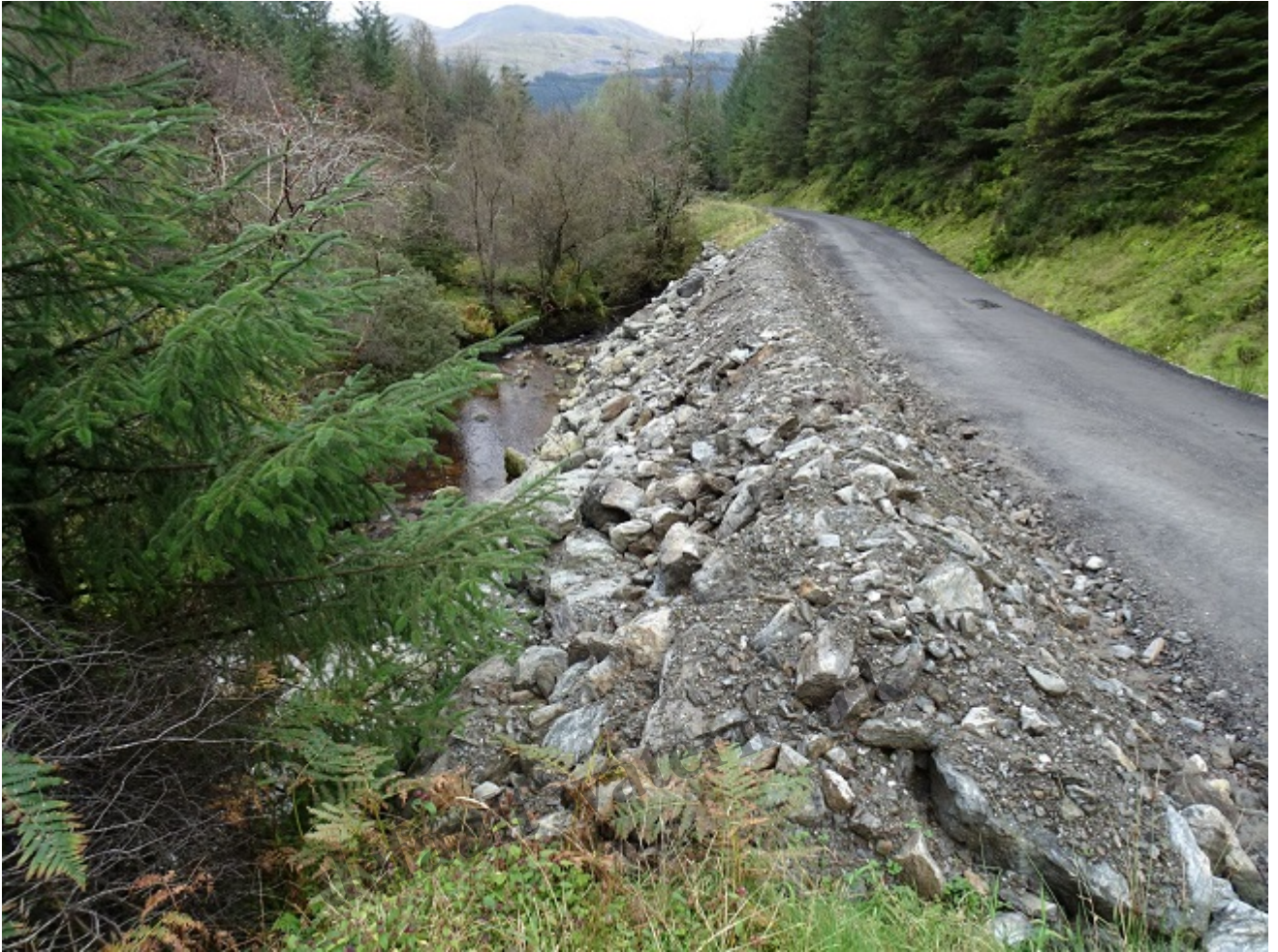
How long before the verge collapses into the burn?
