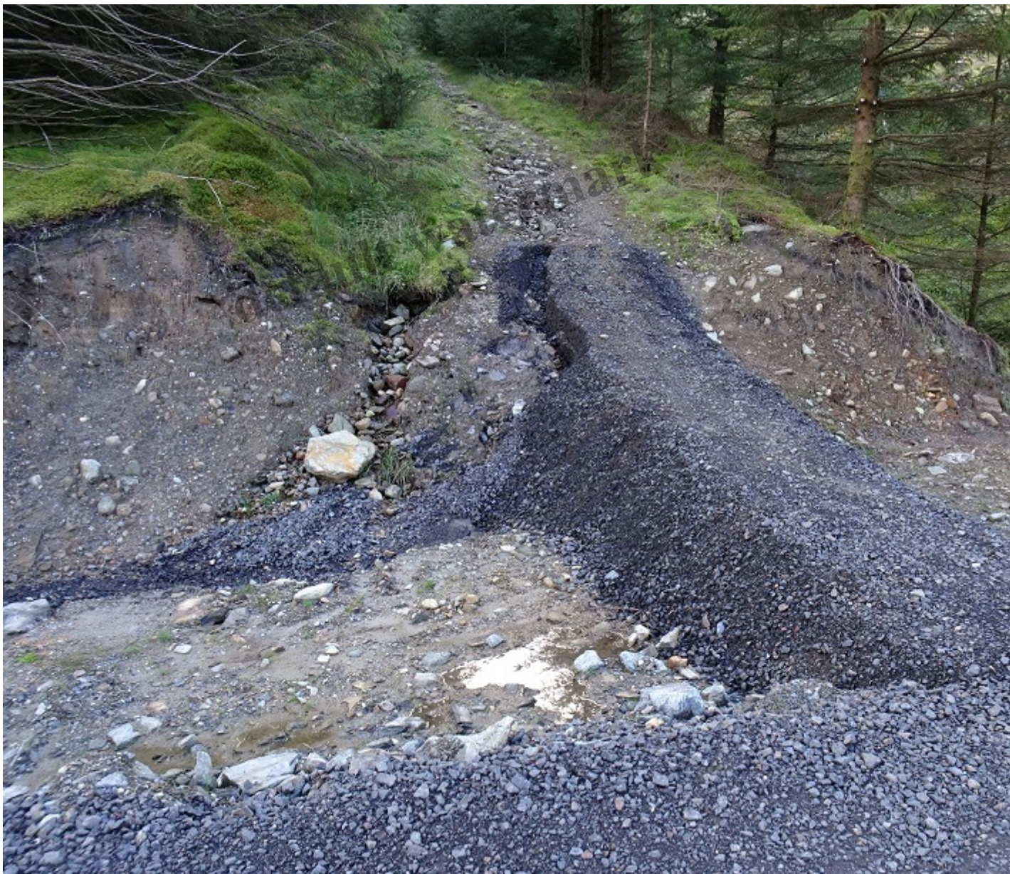
Tastefully designed work in progress at the junction of the Cowal Way with forestry track [Ed. See he of post for how this appeared in April]
