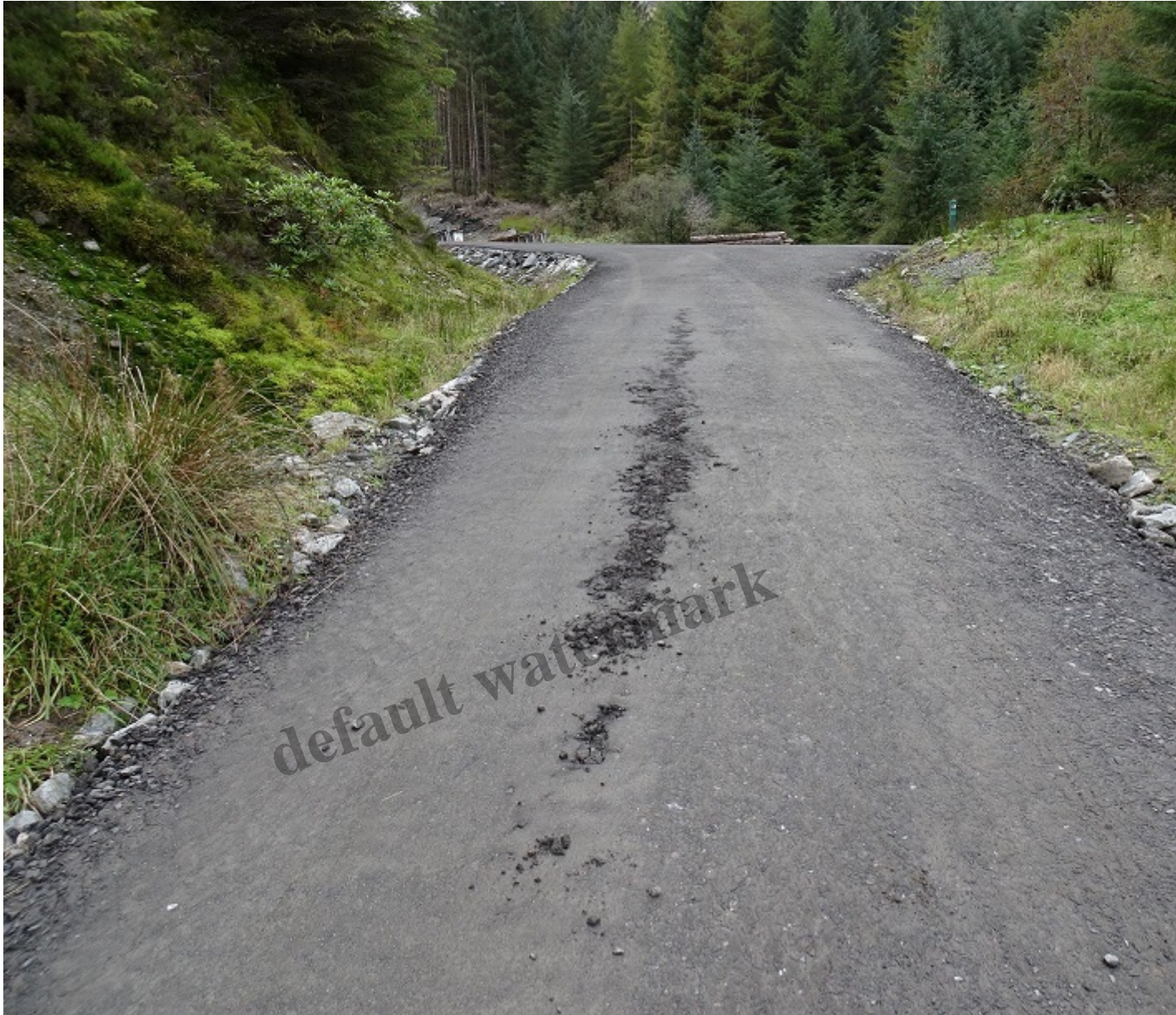
Disintegrating surface finish – one of many examples seen along the way
