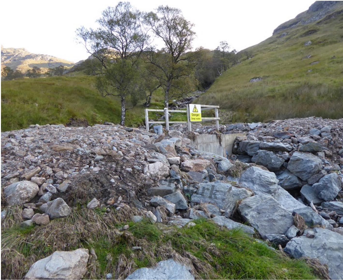
The secondary Allt Chuillinn intake closest to the main intake
