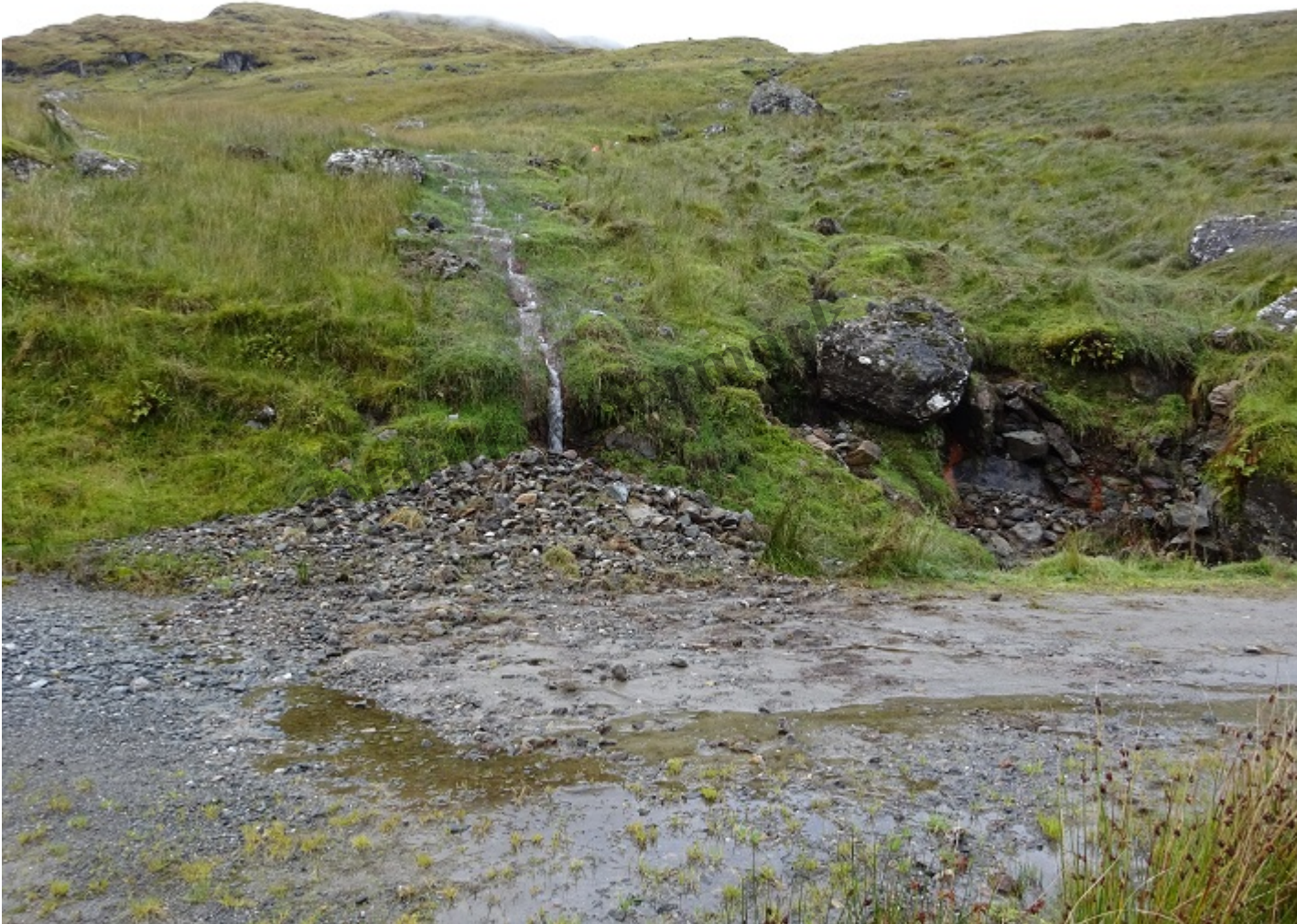
Burn by track up to Upper Glen Falloch hydro intake. Until recently it flowed down by the boulder on right.Â Note the amount of debris washed down by the burn onto the track. Photo credit Kevin McGrath 25th September.
