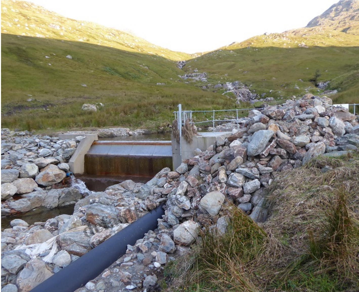
Pile of boulders excavated from pool placed on dam wall – the section of fence behind the boulders intake so the boulders could not have been swept here.
