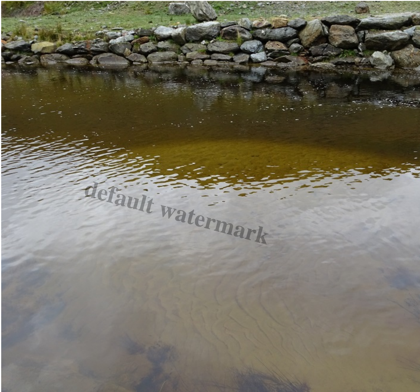
Bottom of intake pool September 2019 – the dam wall is just to the right. Photo Credit Kevin McG
