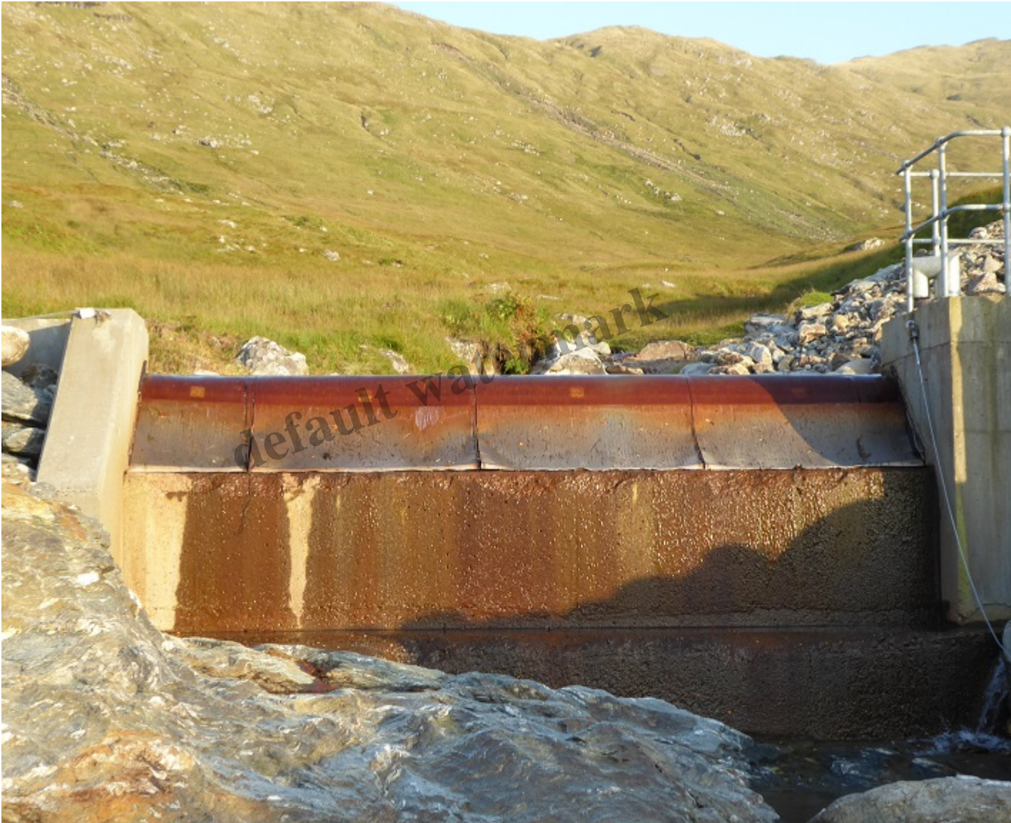
View from below the Allt Andoran intake, part of the Derrydarroch hydro scheme, looking up to the S Garbh – An Caisteal ridge. with a large landslip visible behind extending almost from the ridge to the valley floor.
