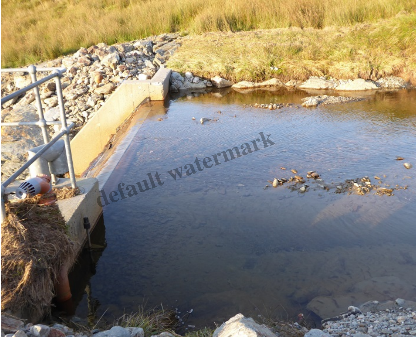
Gravel and silt trapped by the Allt Andoran dam wall. You can see below the lip of the dam a piece of damaged metal from the intake screen sticking up.
