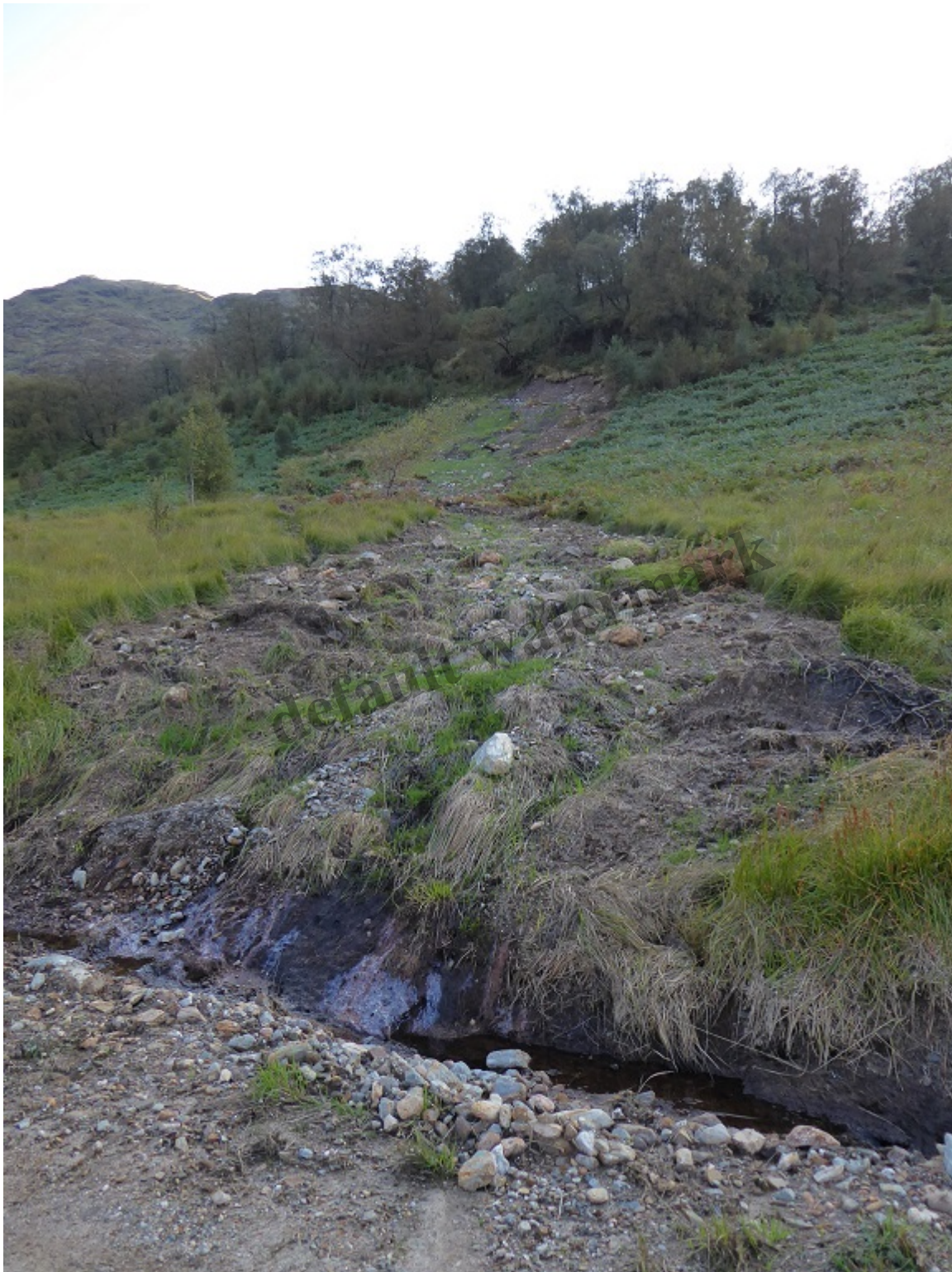
Landslip below Allt a Chuillinn hydro intakes
