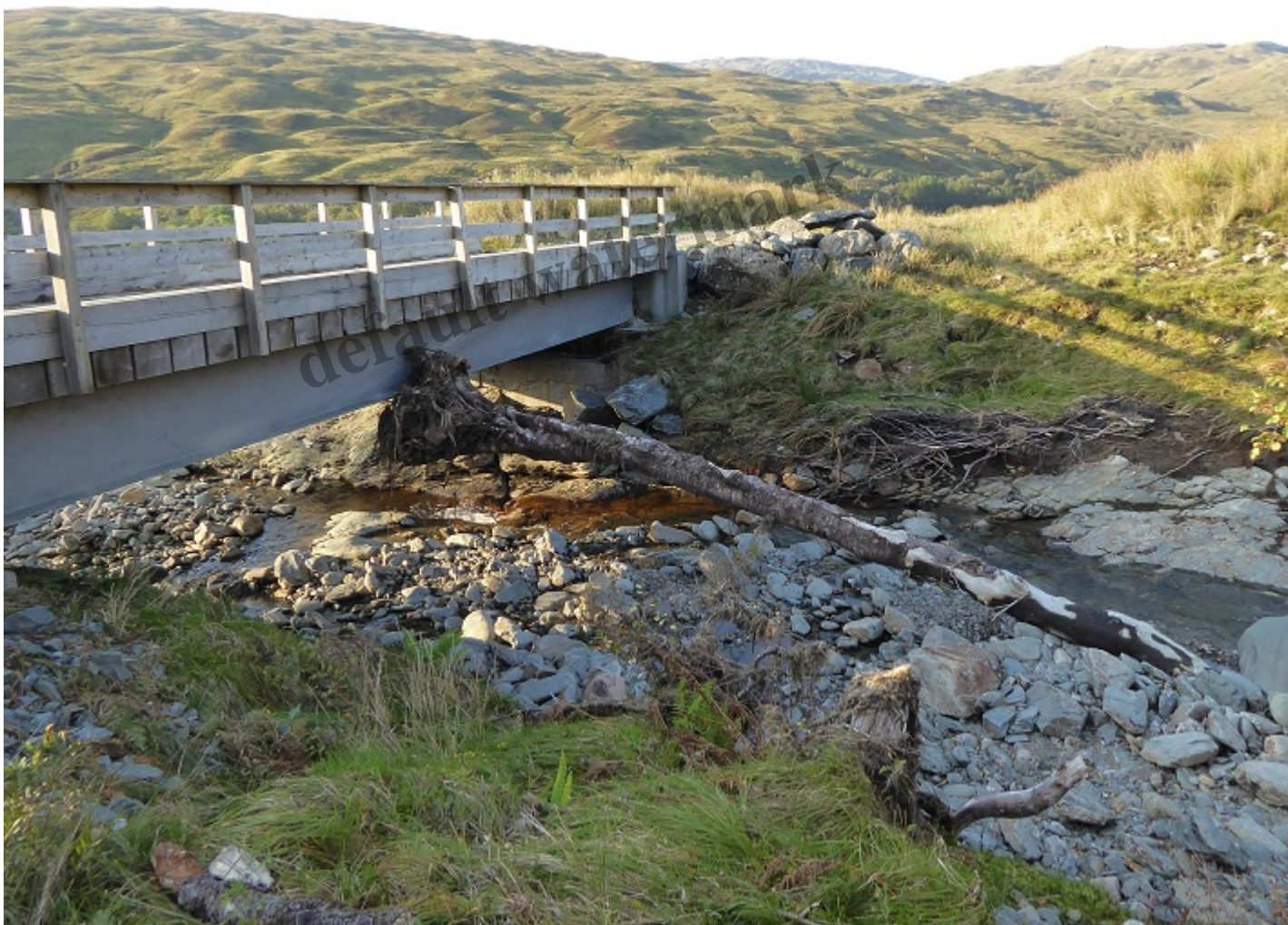
One scene from lower down the Allt a Chuillinn at the new bridge constructed for the hydro scheme. how vegetation has also been removed from the bank on the right
