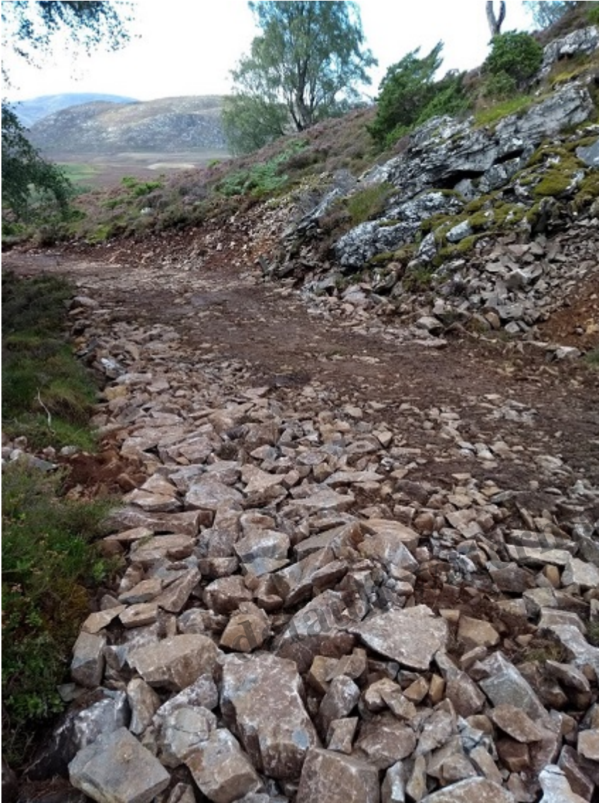
Base of new road being laid with signs of preliminary restoration of cutting on right side of track (stones piled on bank just above centre right of photo)
