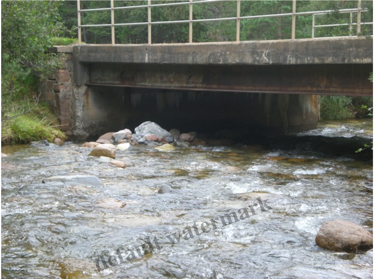
Allt Mhor bridge viewed from above. The flooding has created a new bank of boulders on the opposite side of the bridge to that which was infilled last year. Photo credit Alan Bratney.
