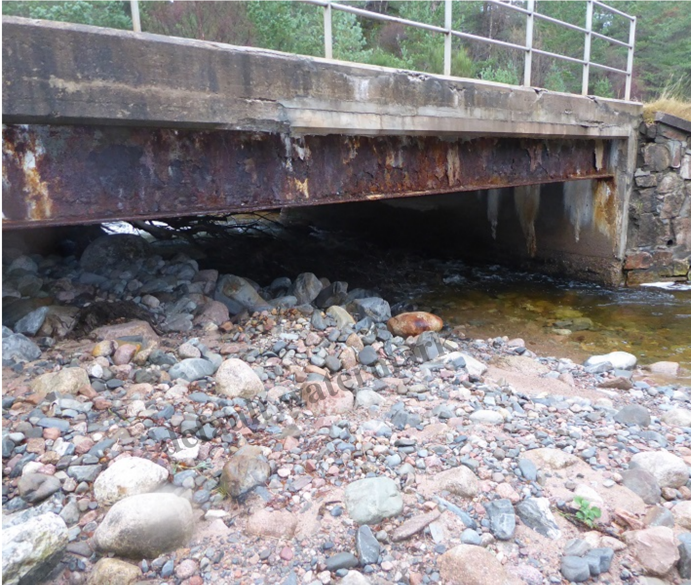
Allt Mhor bridge November – viewed from below – note how the left side of the bridge was half blocked by boulders
