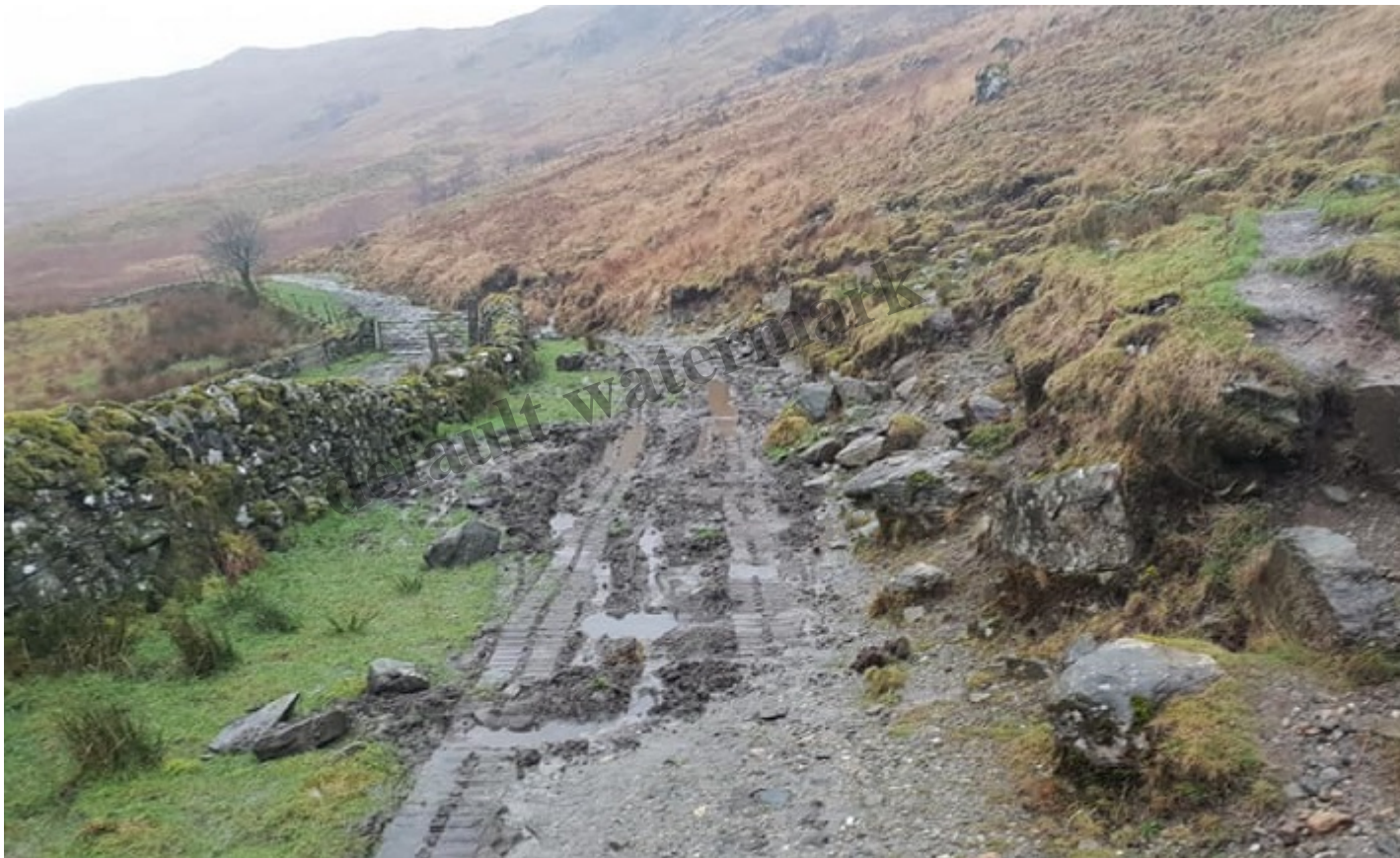
Looking west along West Highland Way to junction with Keilator farm prior to works. Photo credit Gordon Baillie Contracting Ltd
