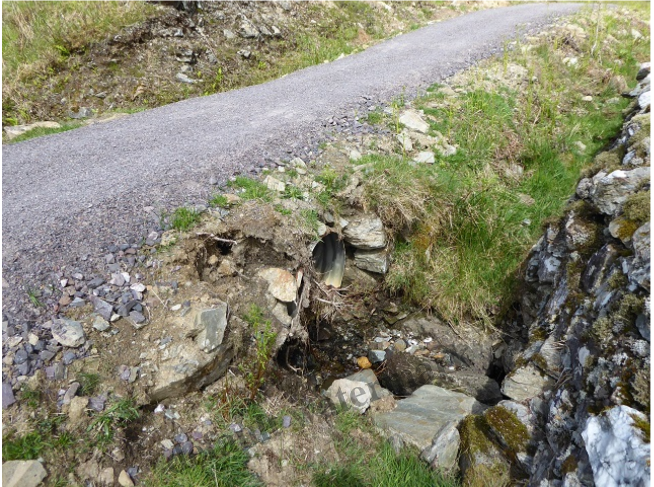
Another collapsing culvert which unless addressed is likely to erode back into the path surface in the near future
