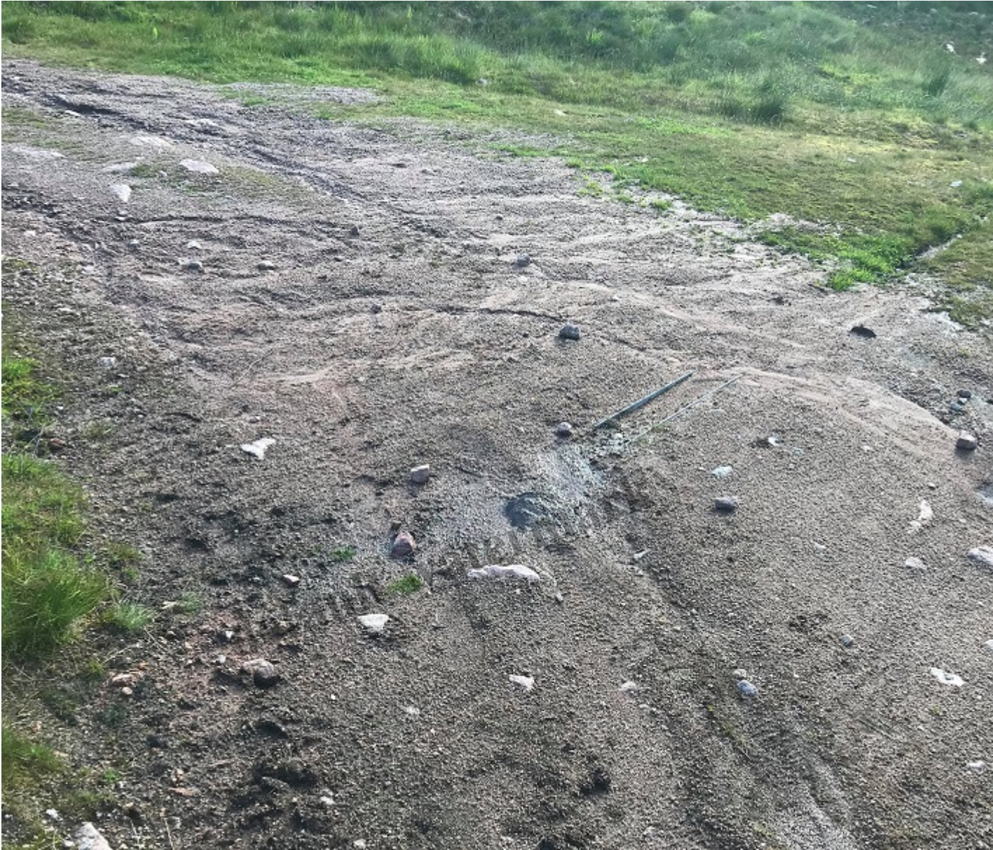
Besides the obvious erosion note the filled in water bar bottom left. Photo courtesy of Alan Bratley.
