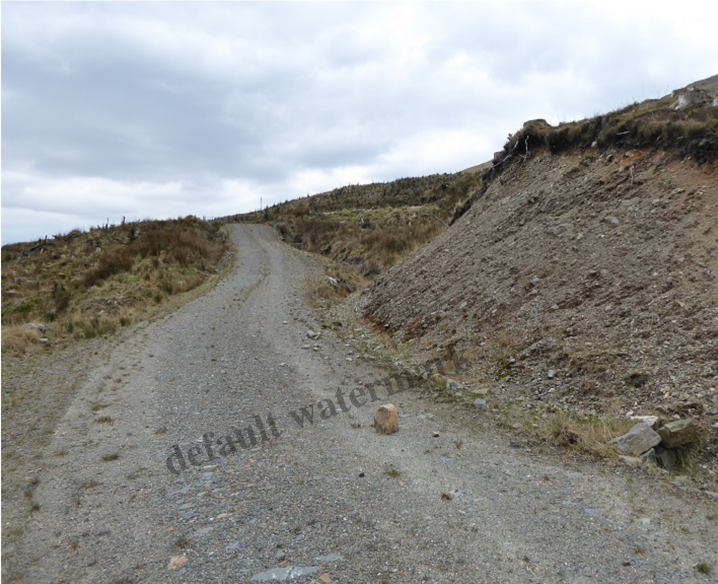
The top spur to the intake – there has been no attempt to restore the bank which is now eroding
