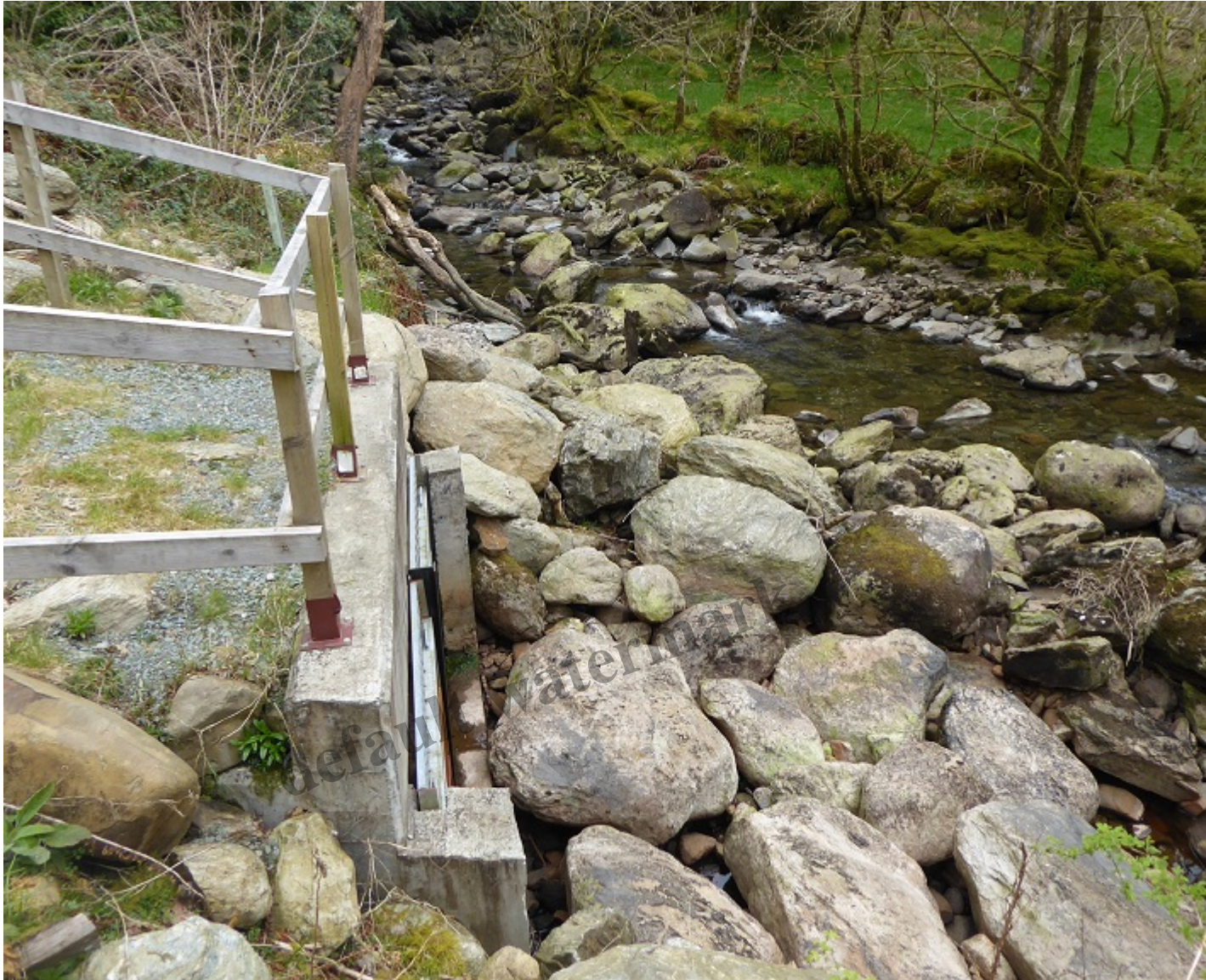
Tailrace – where the water from the powerhouse would re-enter the river if the scheme was operating
