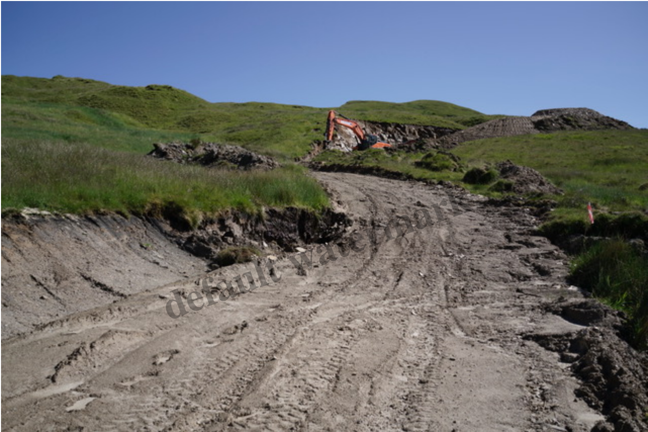
Construction in progress. Note the bare sides to the ditch on the left and the piles of peat and turves on either side of the road. Photo Credit Tom Prentice.
