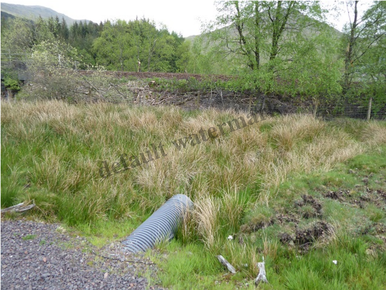
Protruding culvert on new section of footpath between the layby commonly used to access An Caisteal and Beinn a Chroin and the river Falloch
