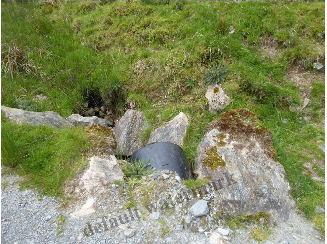
Another collapsed culvert headstone
